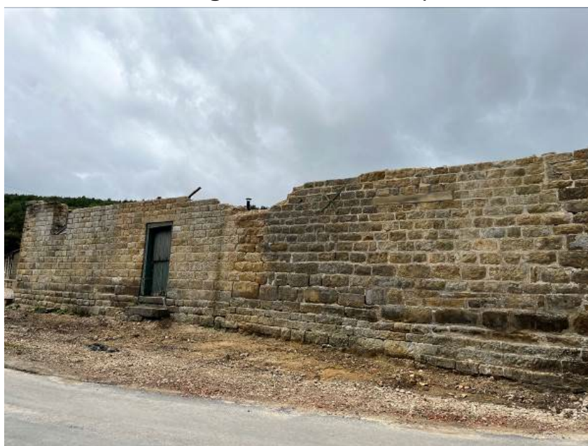
Building now after roof collapse
