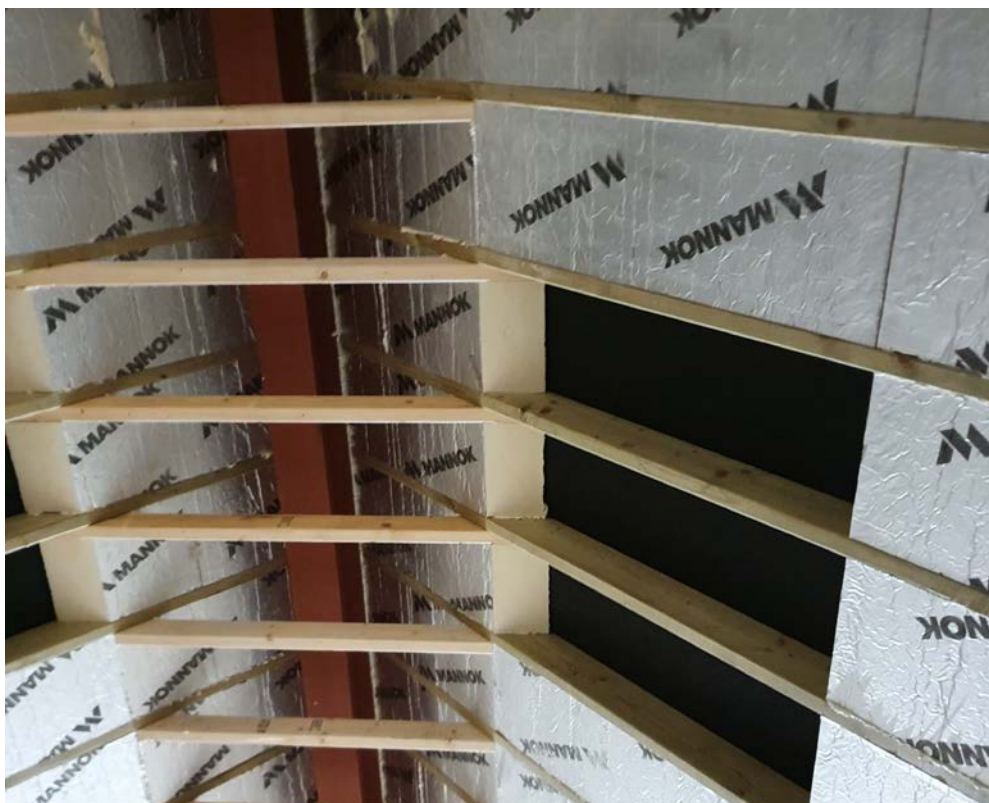
General view of the roof structure with steel ridge beam and timber rafters.
