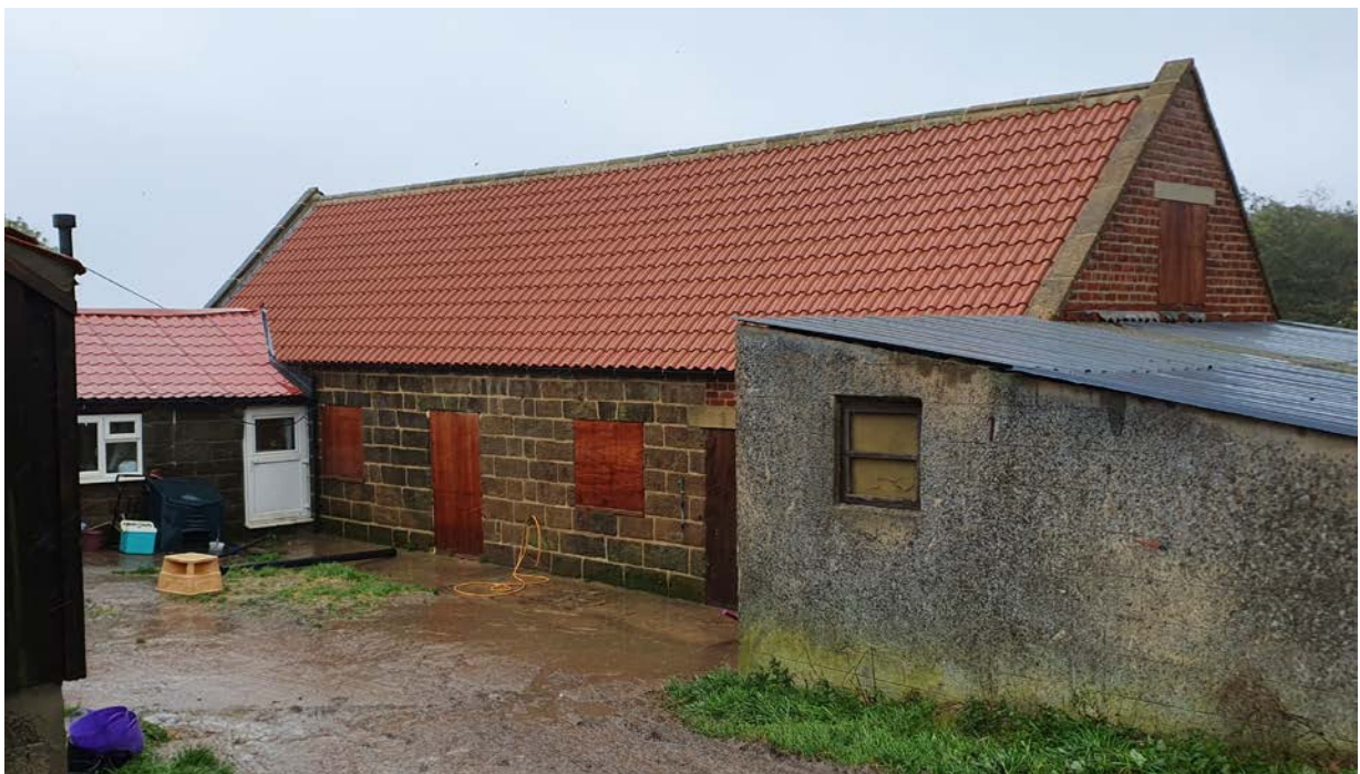
View of the west elevation facing the farm yard with the south brick gable visible over the attached farm shed.
