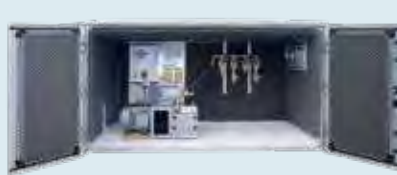
Concrete external cabinet
