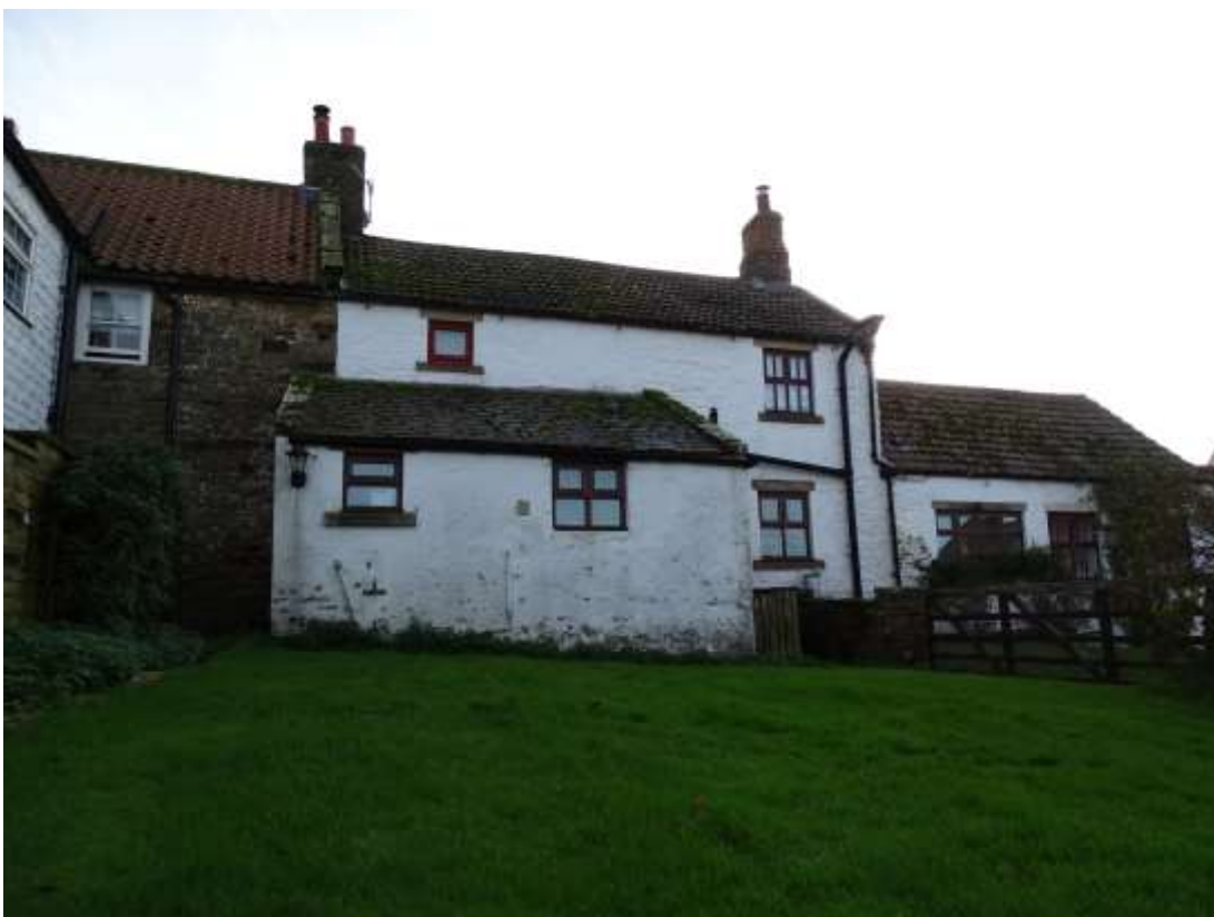
Rear view of the property. Single storey rear extension laps over onto the neighbouring house rear elevation. The rear garden boundary does not line up with the internal dividing/party wall.
