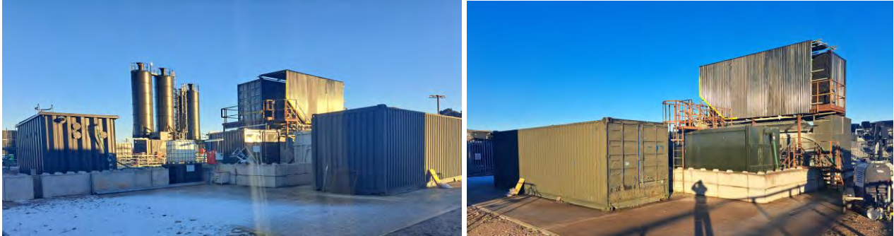
Image 3-2: Lockwood Beck Grout Plant and Filter Press
