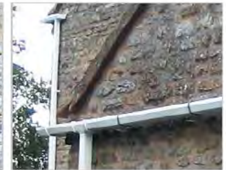
Avoid square section and/or white rainwater goods
