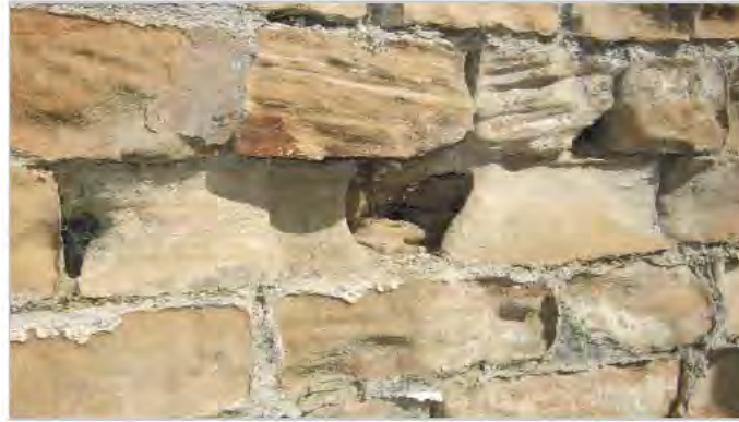
Erosion of the weaker stone
