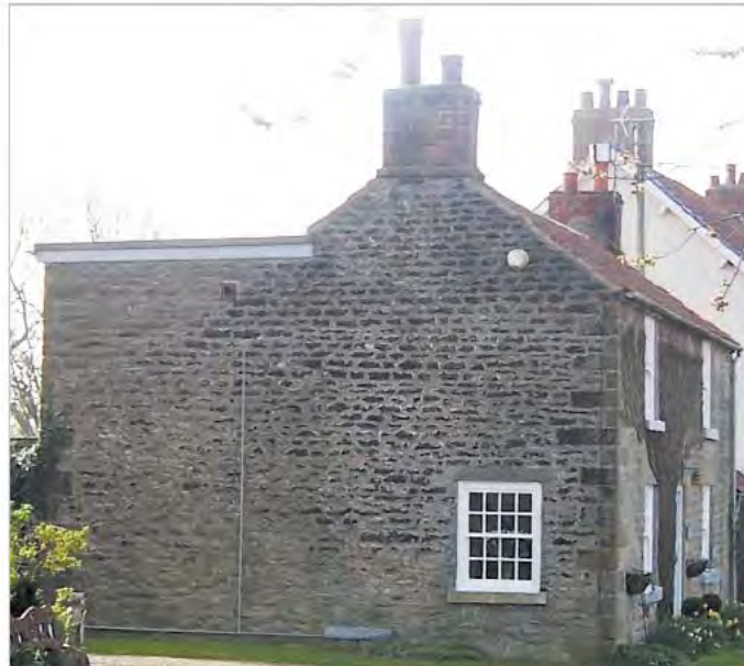
Flat roof extensions can significantly alter the form of the original building and should be avoided
