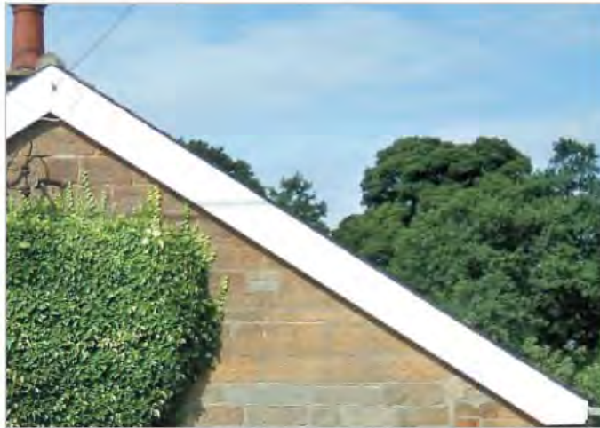
Inappropriate barge board
