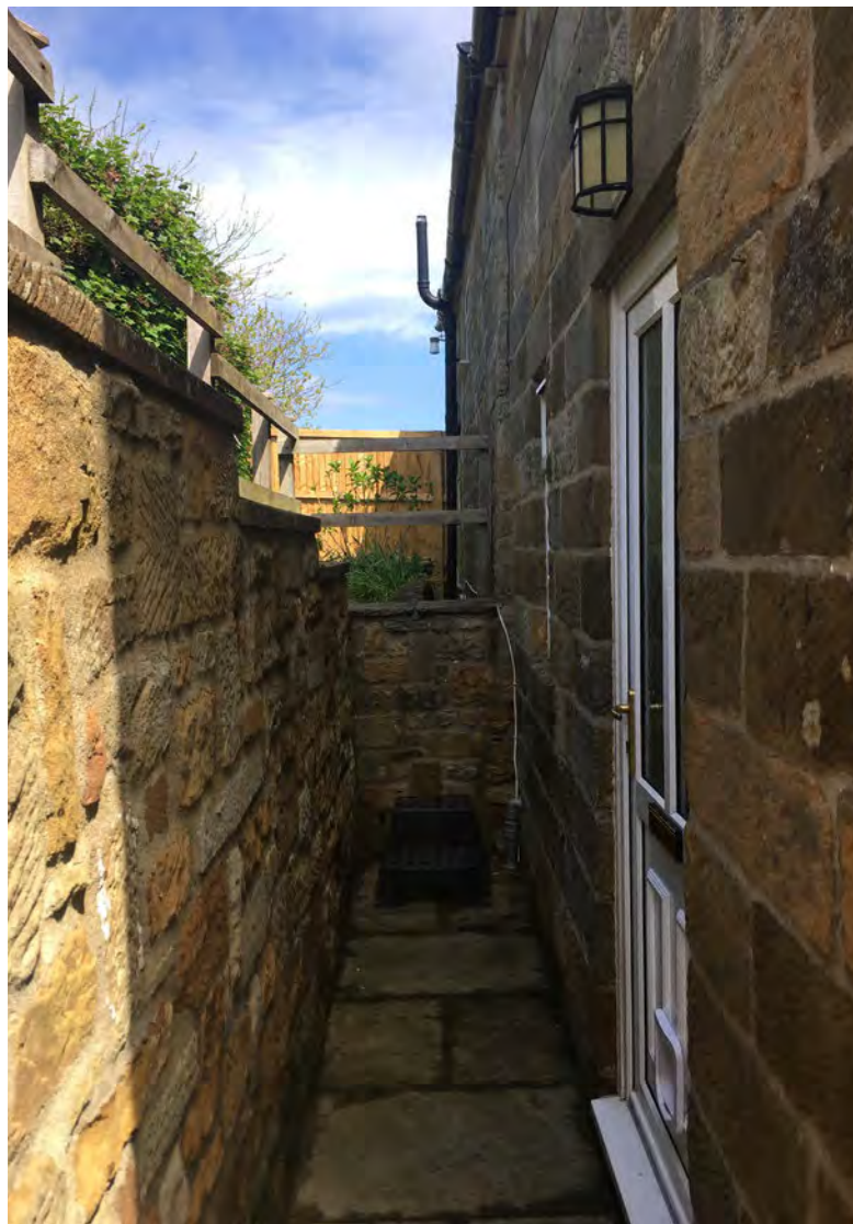
Fig. 26: View looking along the rear elevation showing the retaining wall to the left and the extension approved in 2003 immediately to the right.
