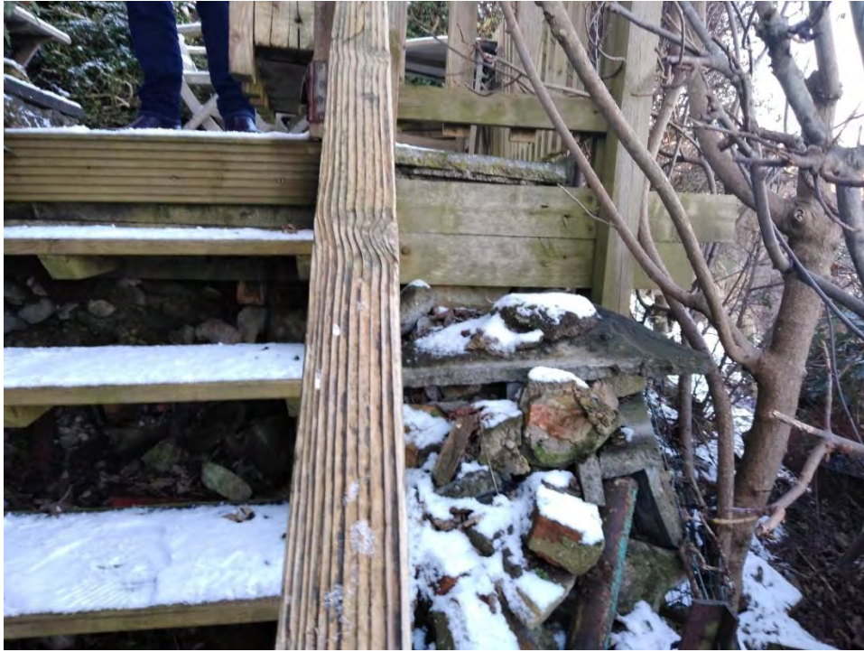
03 View of lower patio showing ad hoc rubble support.
