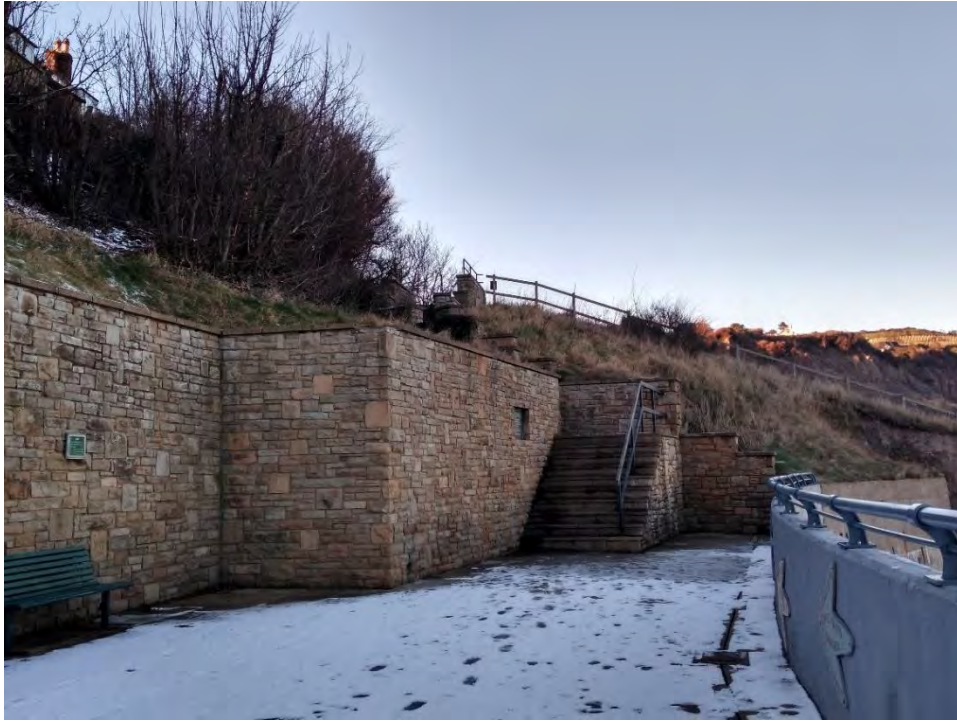
09 View of the stepped access from the coastal slope footpath on to the sea wall (north end).
