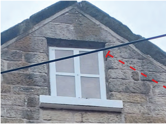
Blocked window to the front
