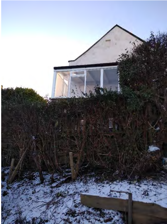
05 View from top of the coastal slope. Vegetation screening to lower patio. Ad hoc supports stabilising surface of the bank.
