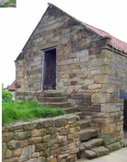
south elevation showing crack referred to in structural engineers report
