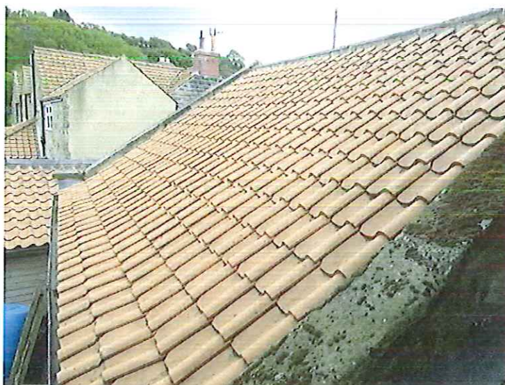
Plate 10 The new roof covering found on the eastern aspect of building 3, viewed from the upper floor of building 2
