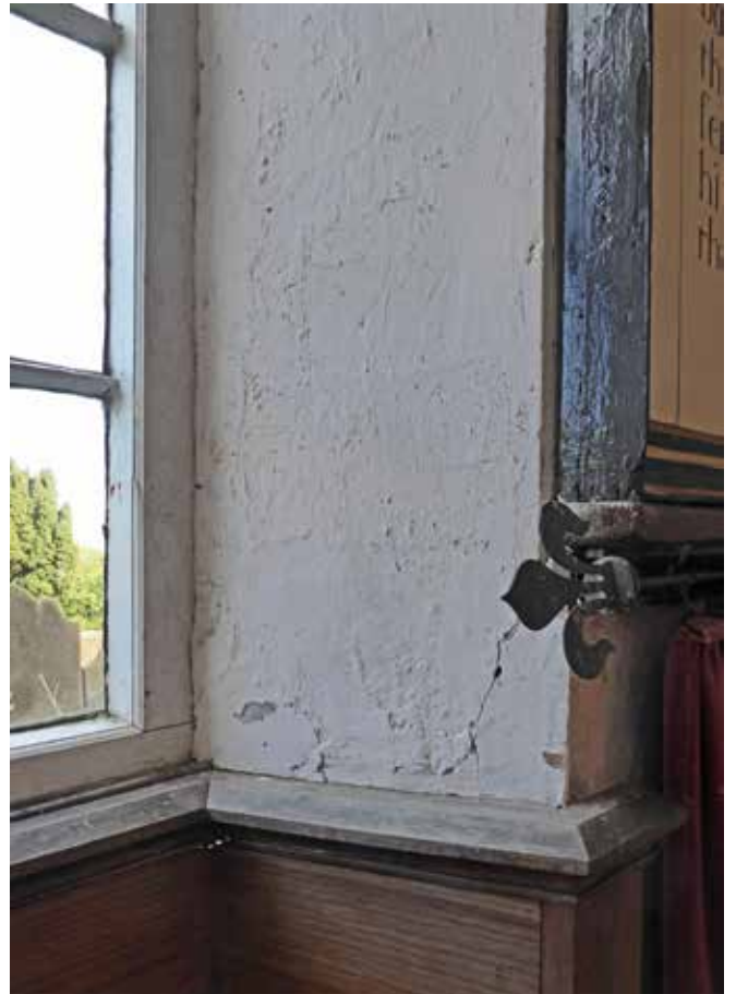
East window, south jamb. Plaster in this area has failed and no longer adhered to the masonry behind.
