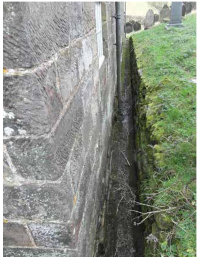
North side of nave - a retaining wall holds back the higher ground level.
