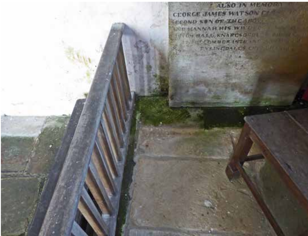
Chancel north side floor. Algal growth indicates high levels of moisture in the floor, not helped by the concrete render and cement floor screed of the vestry behind.
