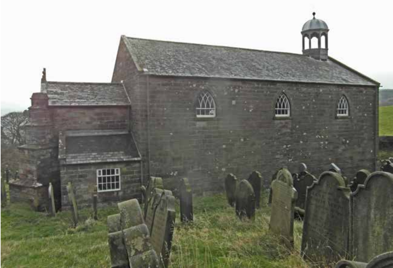
North elevation of nave, chancel and vestry. The ground level on this side is higher than church floor level.
