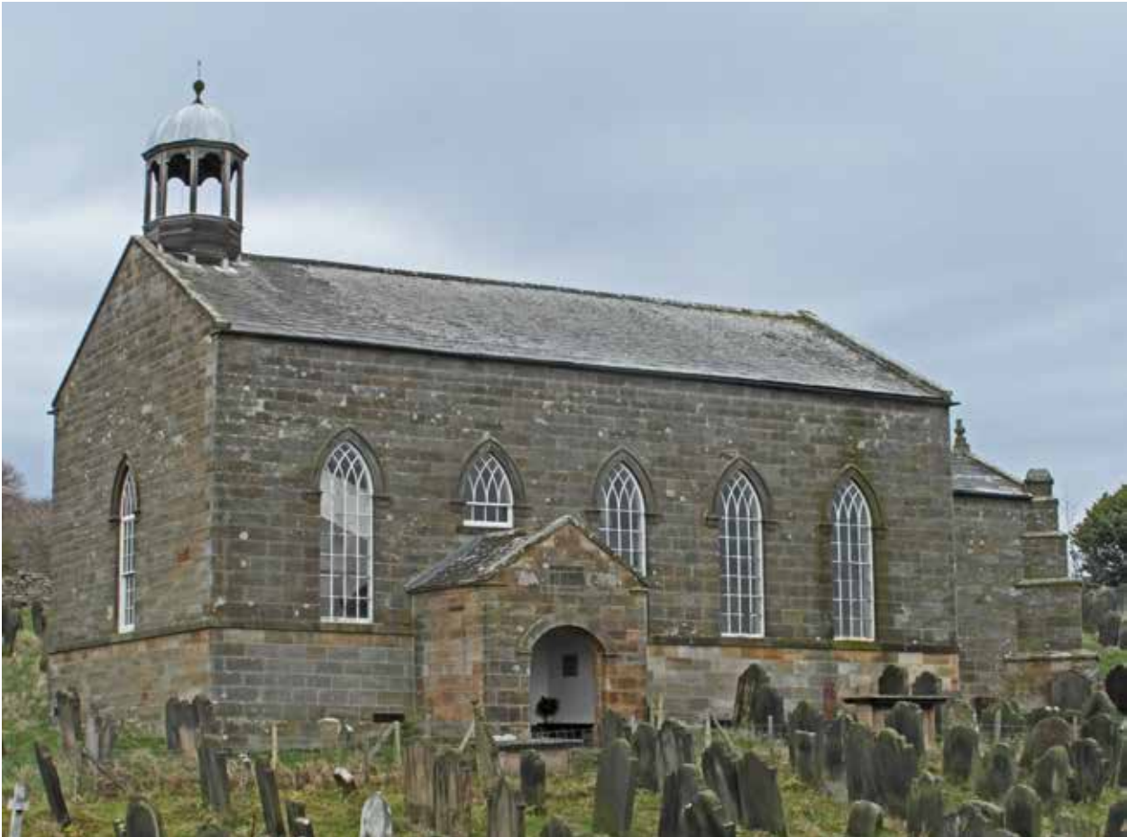
Old St Stephens - south elevation of nave and south porch before redecoration of windows. The churchyard slopes up steeply from south to north and is tightly packed with headstones.
