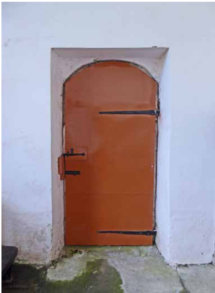
South chancel door. Much of the plaster around this door appears to have been replaced with a hard cement render.
