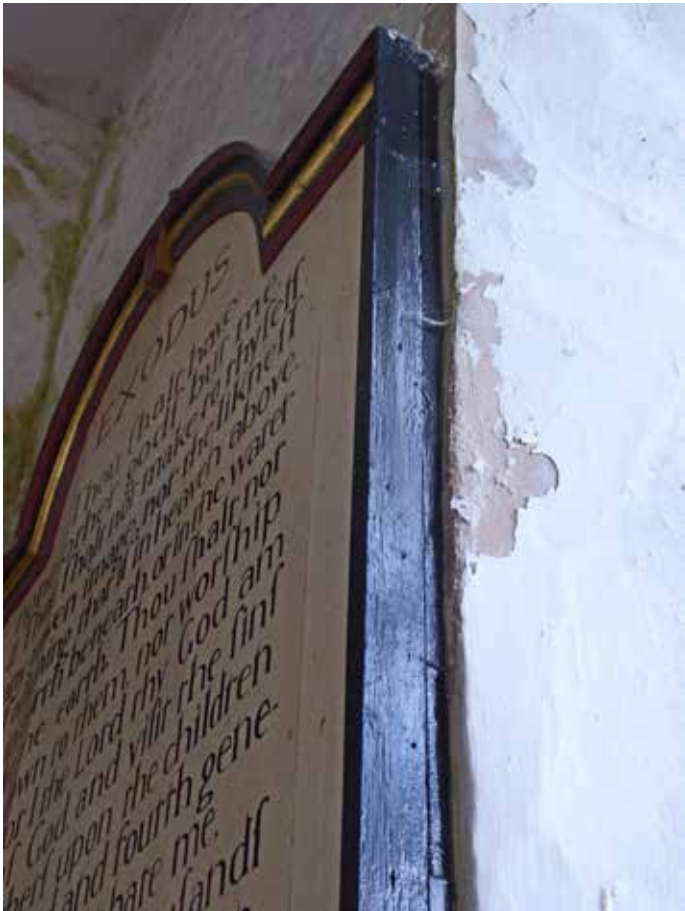
East window, north jamb. Gypsum plaster has been used in a repair. A lack of breathability is causing this to fail again.
