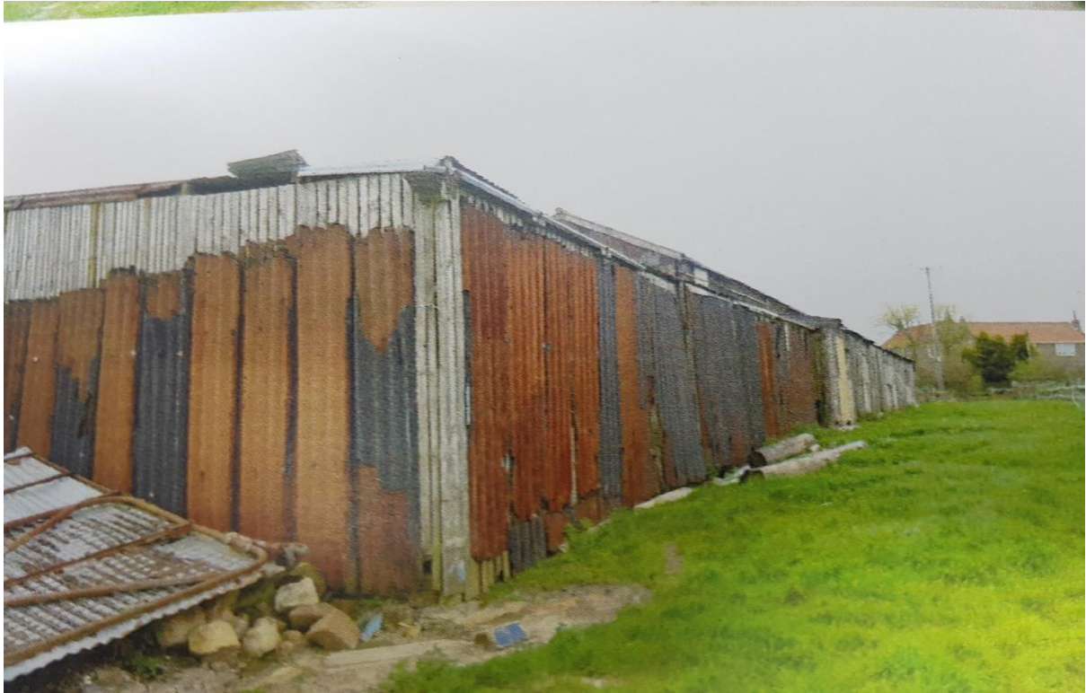
Figure 2. Prior to work commencing on building – black rusty sheeting
