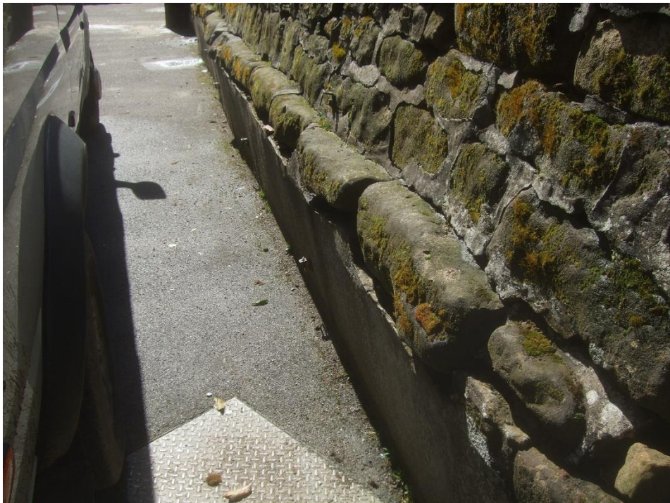
Photograph 3 – outward movement at the base of the wall(recently increased)
