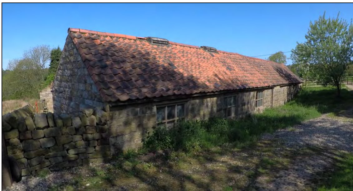
Figure 8: Existing photograph of Barn 2 rear elevation / south side (note: ground level built up against back wall and existing vehicular track passing towards proposed car parking corral beyond)
