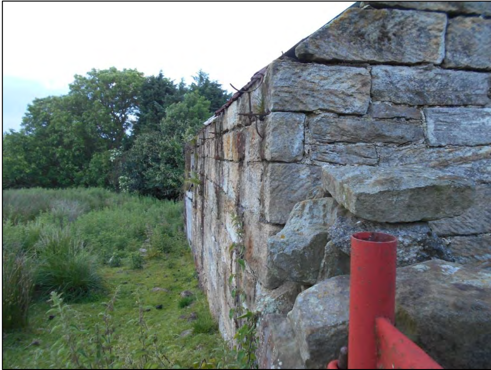
Figure 13: South-west corner showing gaps in exterior pointing
