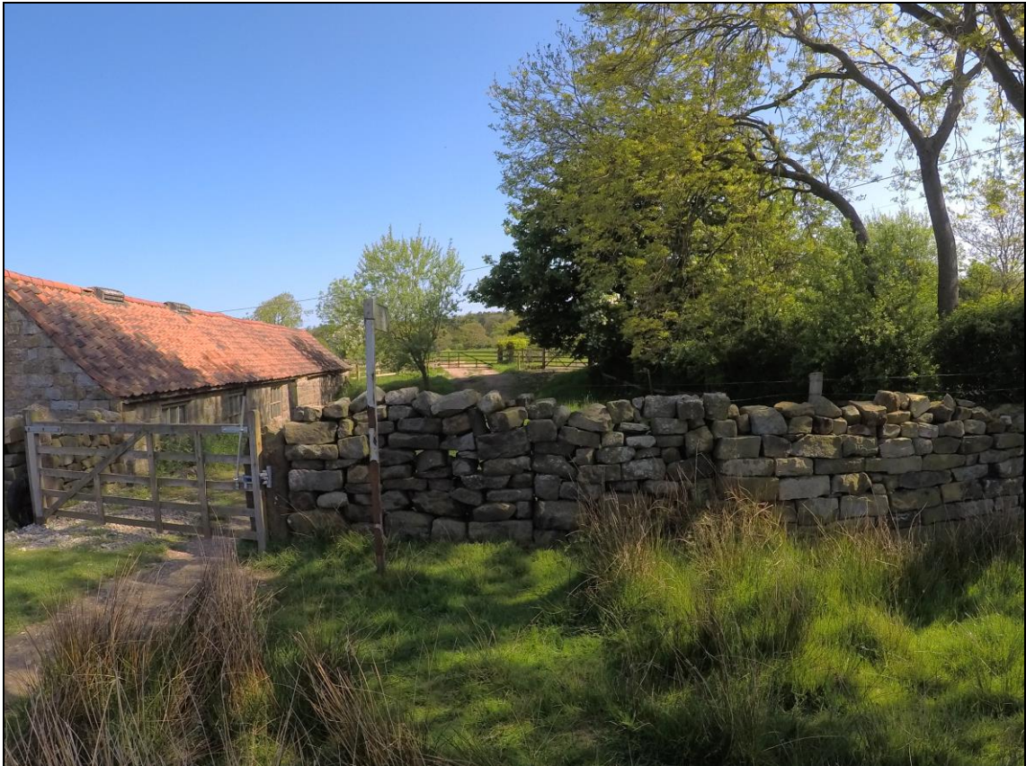
Figure 20: Existing gated access to south of Barn 2. Concrete post can be seen to left hand side; stone post to the right has cut, dressed face to right hand side, indicating it previously would have stood as the left hand post...furthermore, two stages of infill of a previous opening can be seen in the stonework to the right
