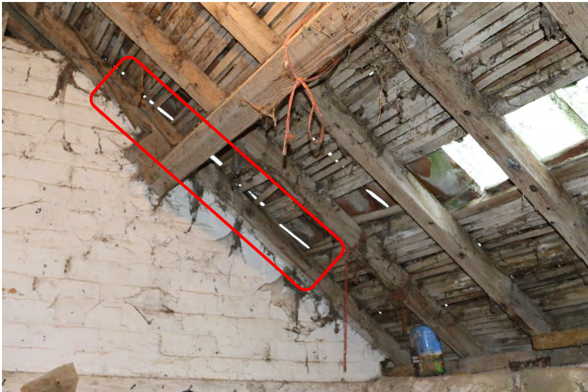
Image 9 – Further views from below the roof coverings within the building in which daylight can be seen above the stonework's
