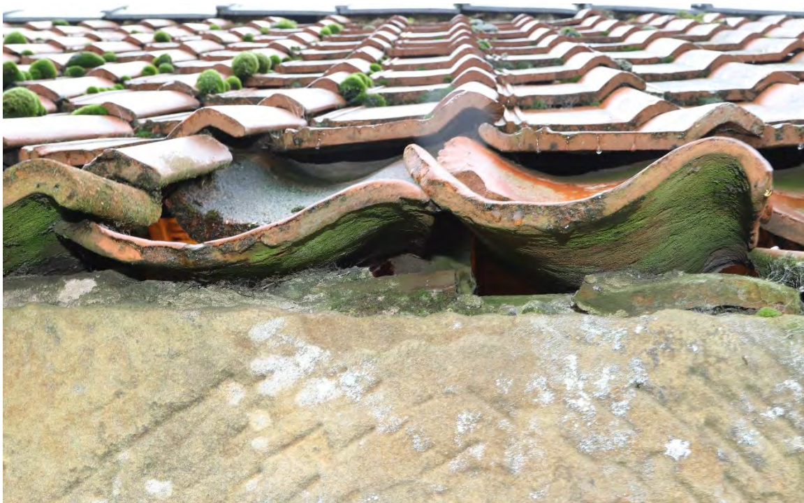
Image 4 – North/West facing roof coverings which offer value to bats with access into the internal areas of the building
