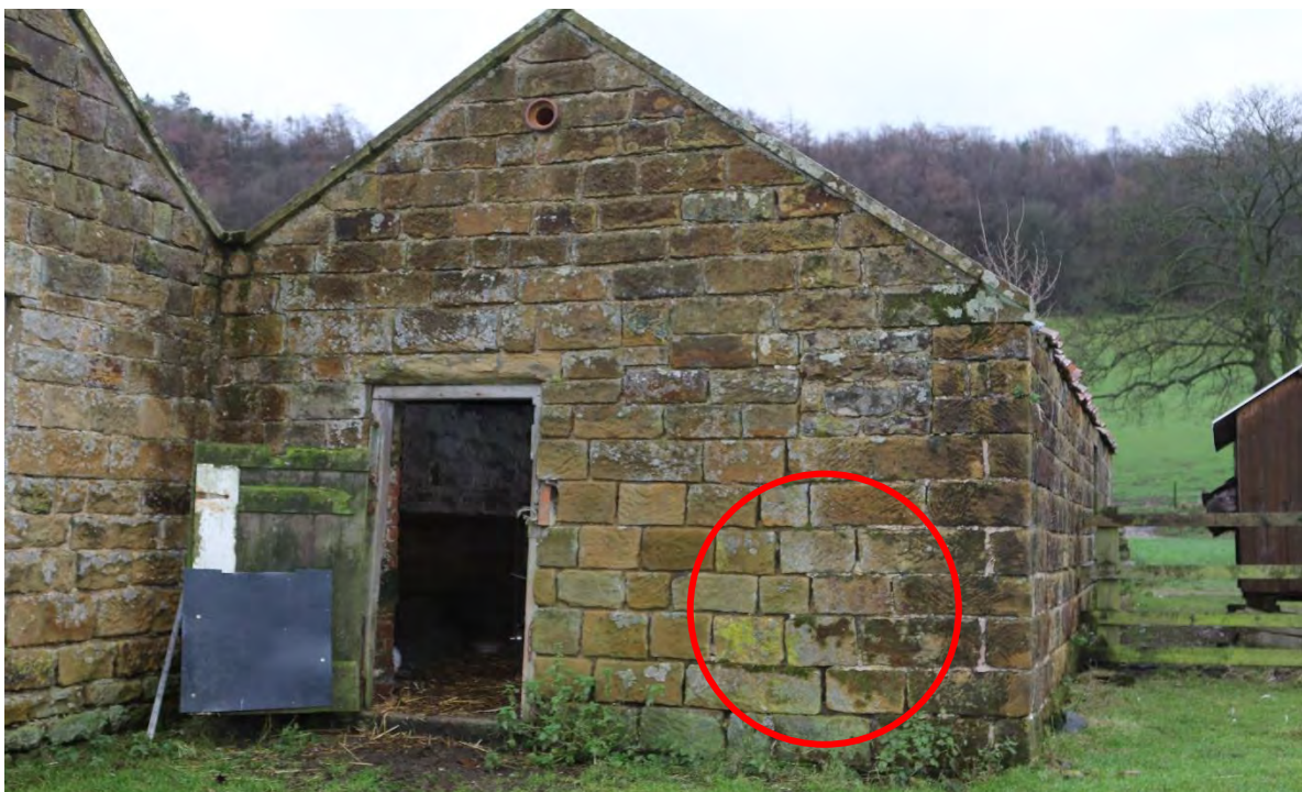
Image 6 – North/East facing elevation of the building in which deterioration has been noted within the stonework's which offer suitable roosting values for crevice dwelling bats within
