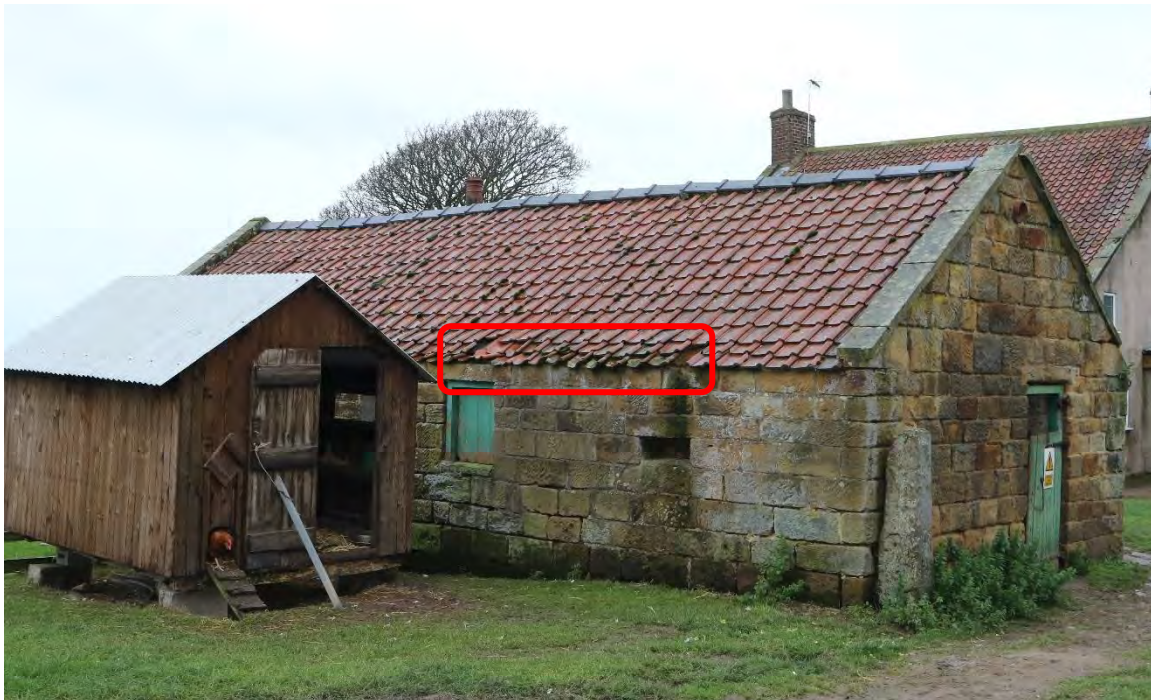
Image 3 – North/West facing elevation of the building demonstrating areas of deterioration/damage to the roof coverings
