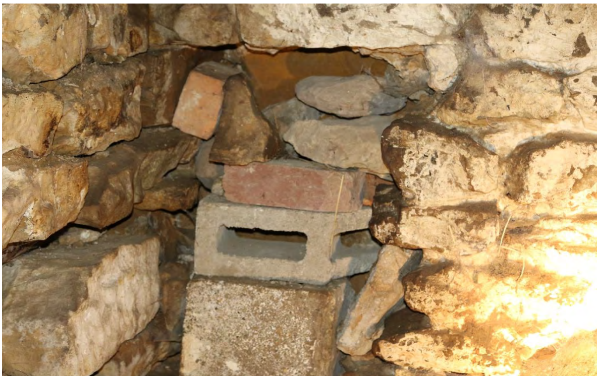
Image 10 – Internal stonework's within the far East area of the building in which a number of suitable roosting areas for crevice dwelling bats have been noted where areas have been patched up and deterioration.
