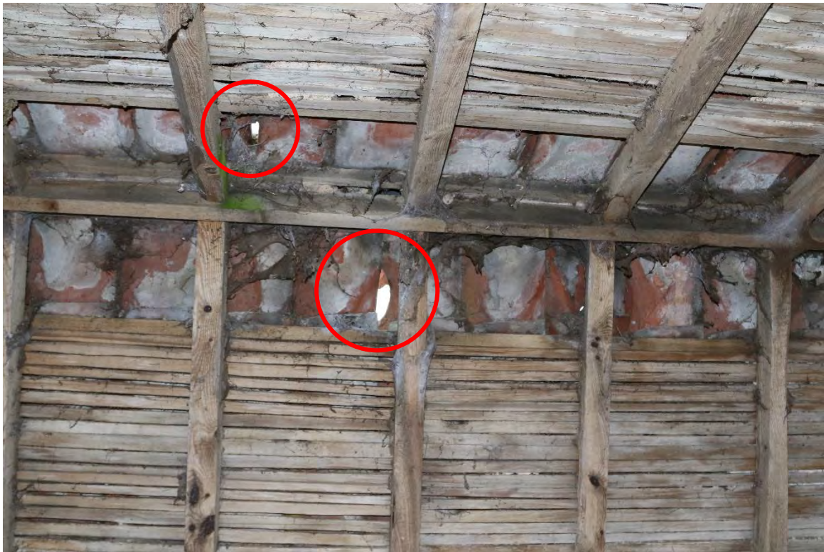
Image 7 – Below the roof coverings where a number of gaps within the coverings of ample size for bats have been identified, also additional timber coverings below
