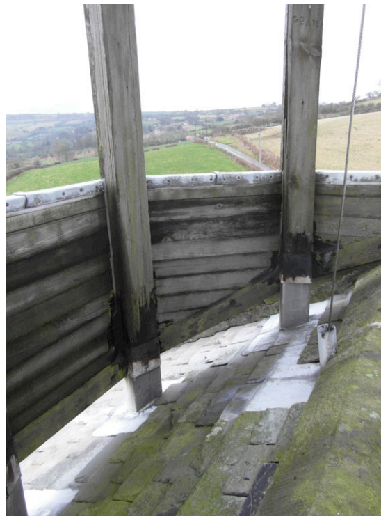
Inside the cupola . The posts continue through the roof with a lead flashing. Water appears to be running down the posts, behind this flashing and down into the roof space.
