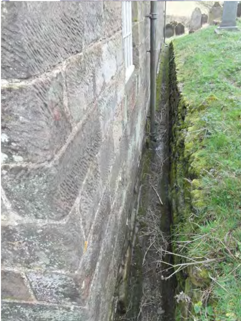
North elevation of vestry and nave. A retaining wall and channel arrangement should direct water to a gully at the west end to discharge to the west of the church.
