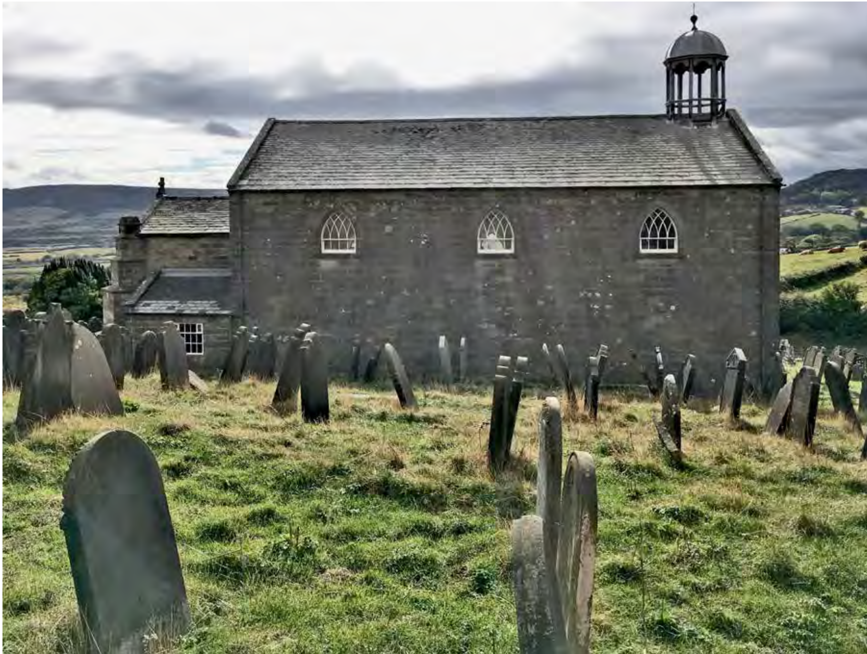
North elevation - the nave gutter drains to a downpipe at each end before being channelled to a gully at the west end of the church. Proposals involve removal of the east (left downpipe). On the south side of the church there is a single downpipe at the east end.
