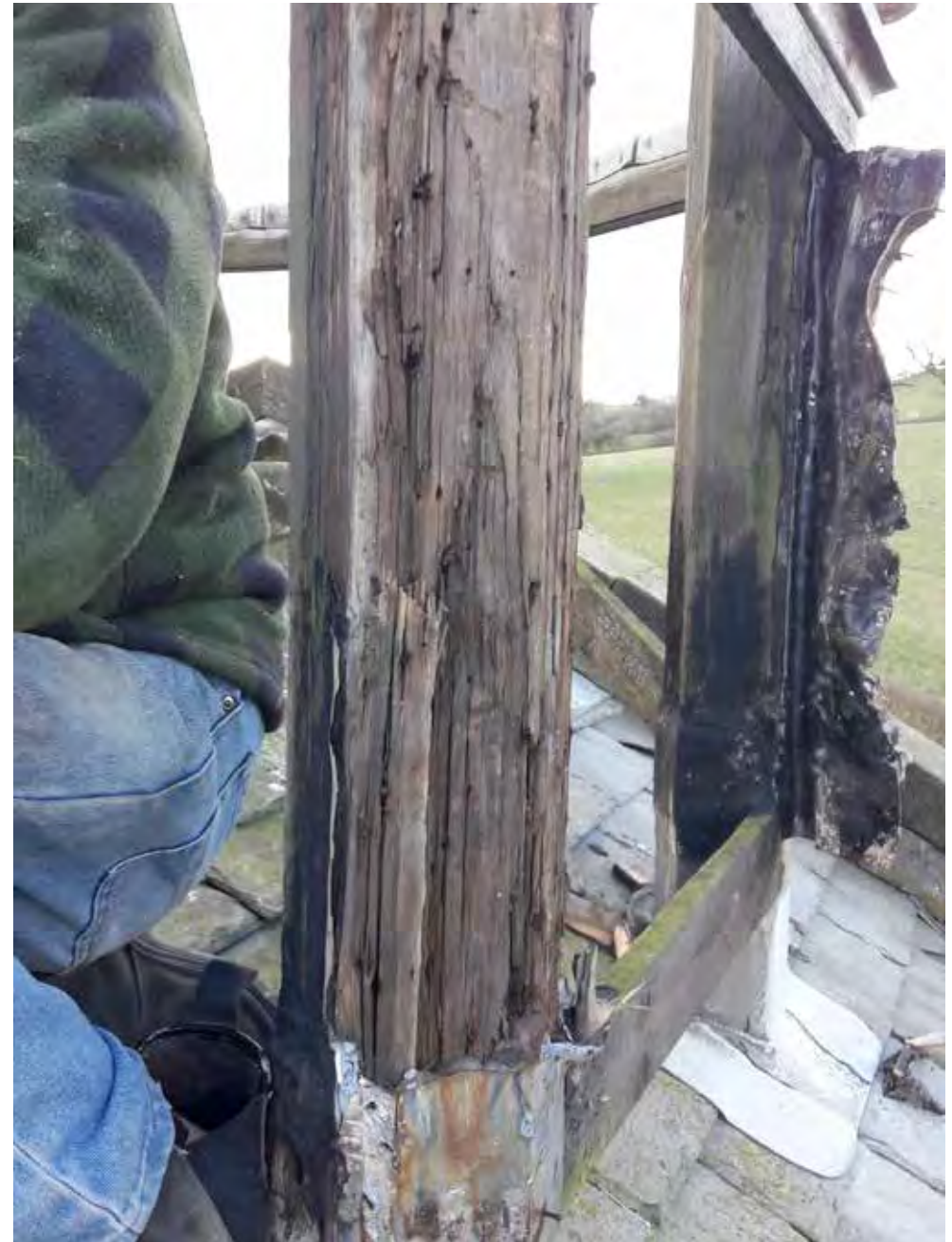
Behind the boarding there is quite a bit of decay in the timber support posts.
