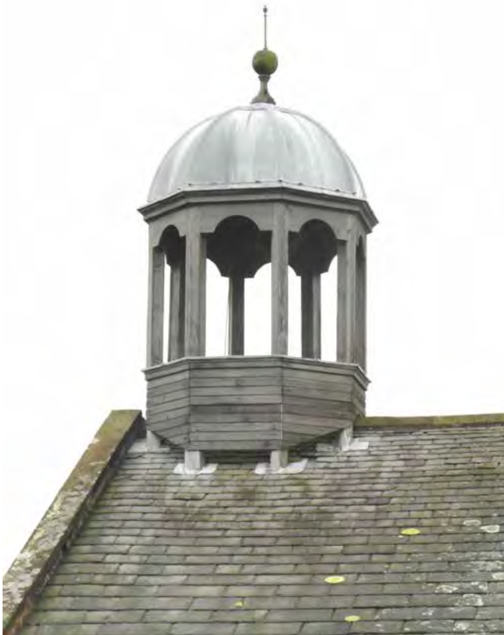
Existing cupola, before investigation of water leaks and removal of horizontal boarding.
