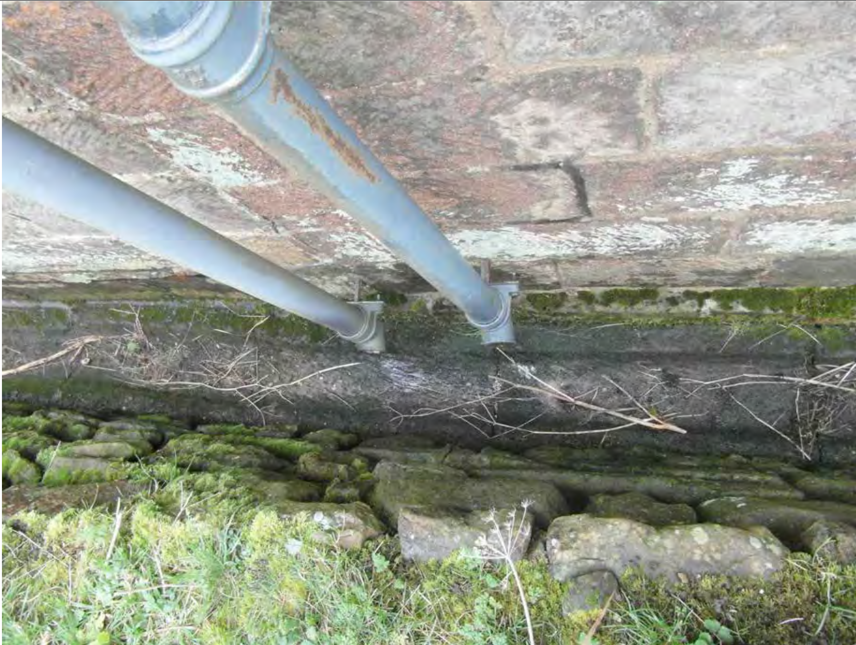
Downpipes from the vestry and nave discharging on to the channel at the foot of the north wall. While little can easily be done to redirect water from the vestry roof the nave gutter can be adjusted to discharge to the west downpipe only.
