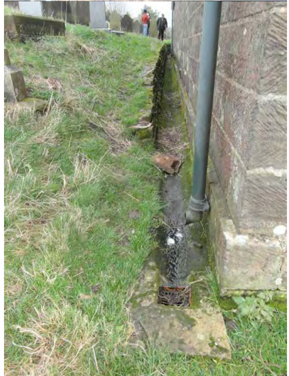
Unfortunately debris, open joints and mis-aligned channel stones allow much of the rainwater to drain into the ground, under the church.
