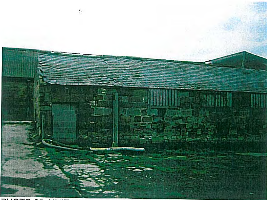
PHOTO 25. UNIT 10 – LEFT HAND SIDE ELEVATION
