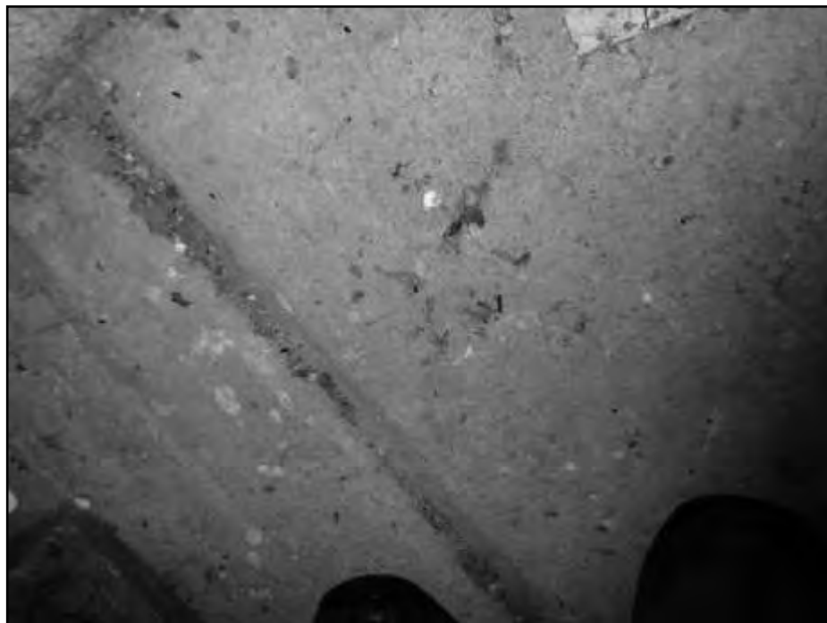
Figure 41. Bat droppings present on the ground floor
