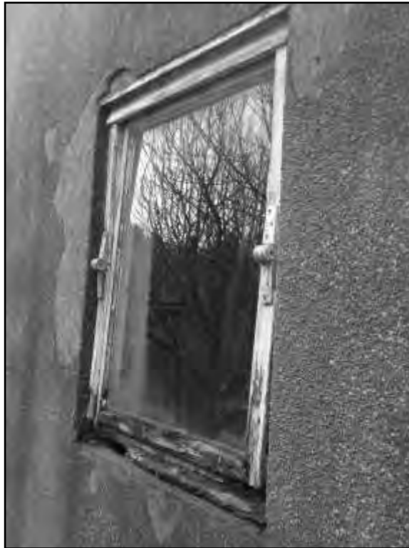
Figure 20. Window frames are rotten and in a poor state of repair
