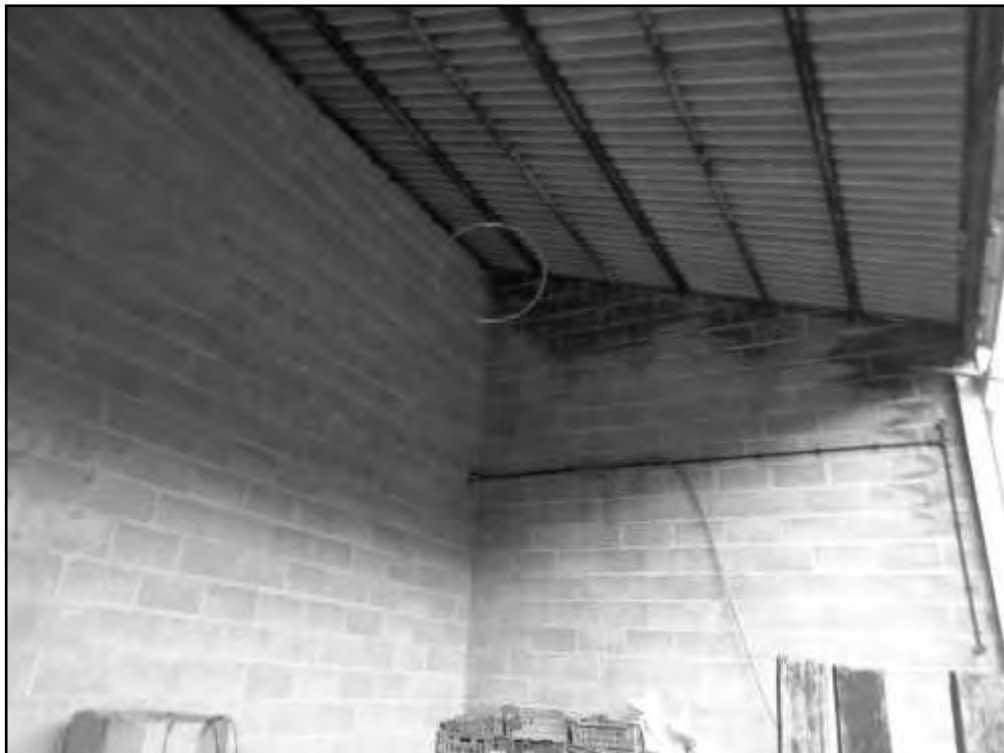
Figure 33. Open barn on south eastern elevation. Remnant bird's nest and potential bat roost entrance marked
