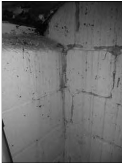
Figure 31. Bat droppings scattered across the first floor – on the floor, walls and wall tops
