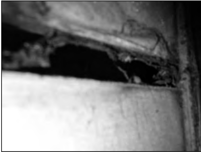
Figure 28. Gaps present in the ceiling below the asbestos sheeting
