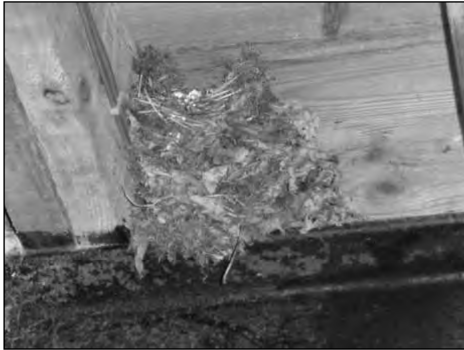
Figure 40. Remnant bird's nest on the ground floor (TN9)
