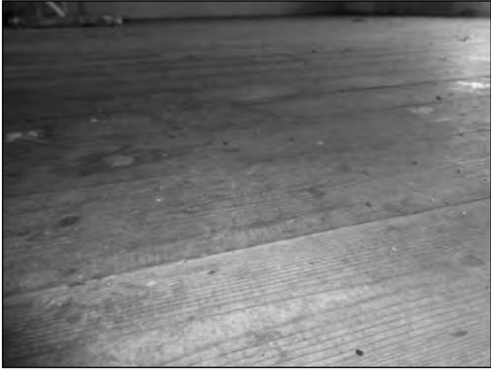
Figure 32. Figure 31. Bat droppings scattered across the first floor – on the floor, walls and wall tops
