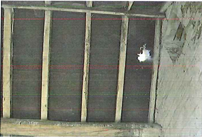
Photo 19: Hole in sarking and aperture through to adjacent room.
