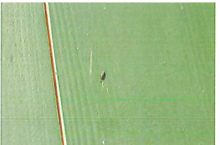
Photo 32: Bat dropping on door 4.
