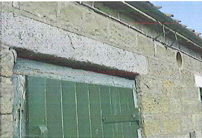
Photo 6: Gaps above doorframe
