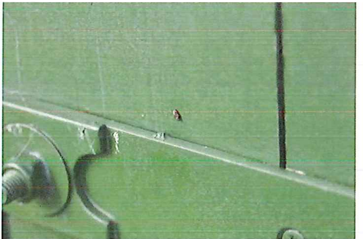
Photo 30: Bat dropping on door 3
