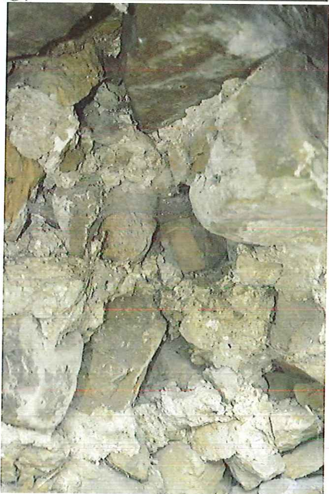
Photo 11: Collapsed area of wall
