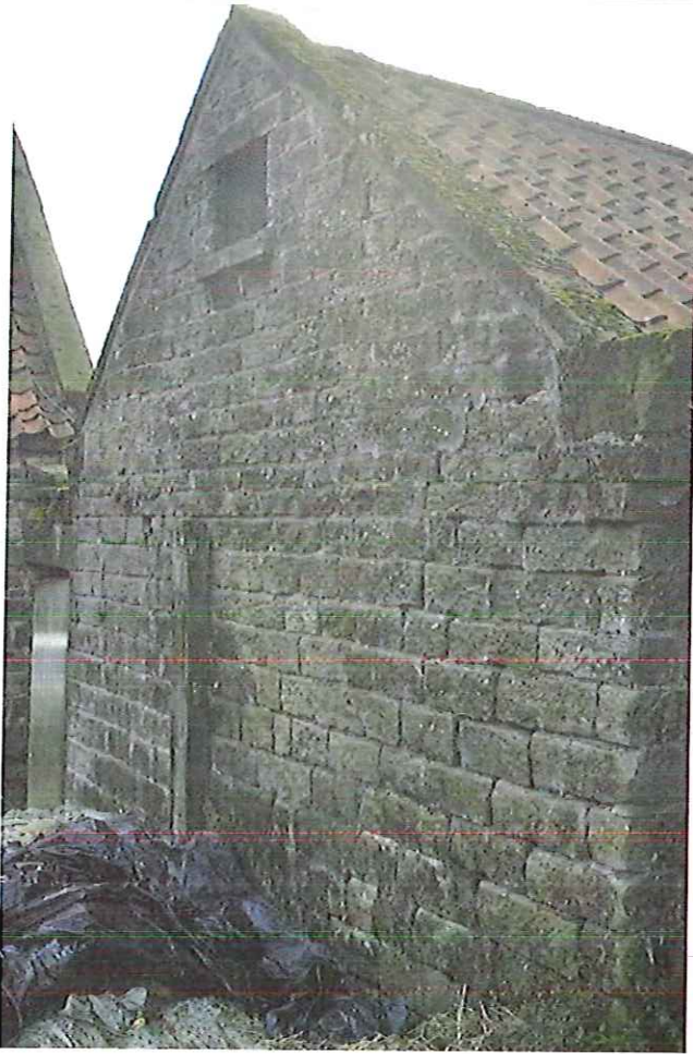
Photo 10: Poor condition of gable end wall
