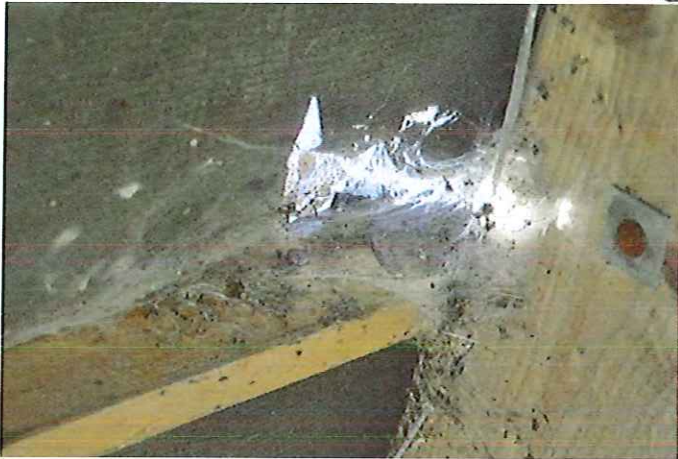
Photo 17: Hole in sarking
