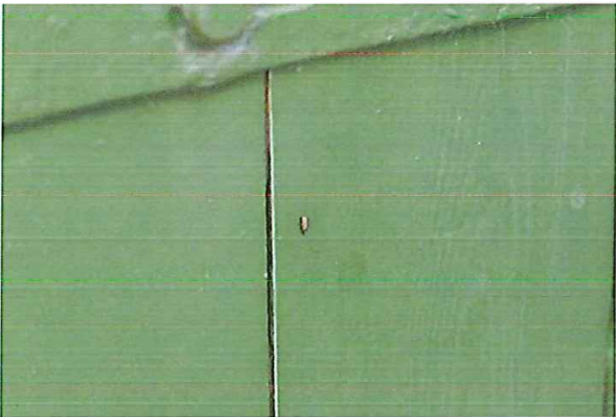
Photo 29: Bat Dropping on door 2
