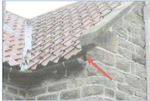
Photo 6 - Gap at corner at eaves level.
