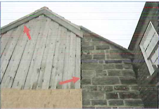
Photo 7 - Timber fascia and cladding to western gable, with crevices between timbers and stone work.
