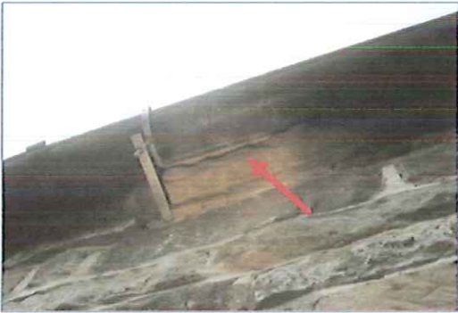
Photo 5 - Gaps along eaves on eastern elevation.
