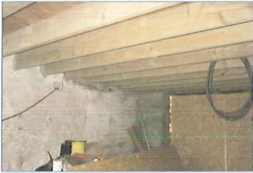
Photo 3 - Upper floor timbers. Crevices are present where timbers meet the internal walls.
