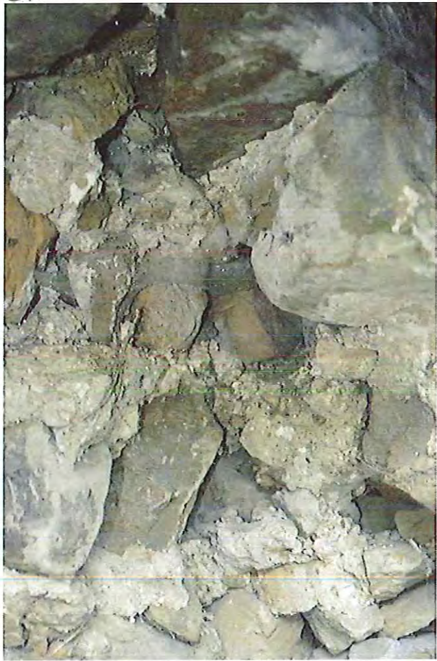
Photo 10: Collapsed area of wall
