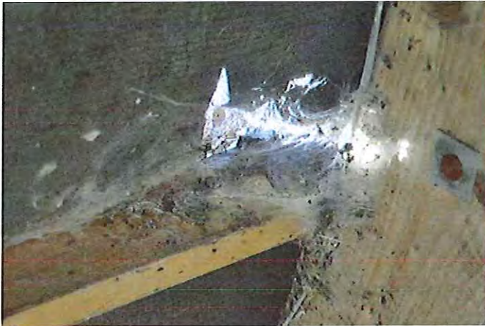
Photo 16: Hole in sarking
