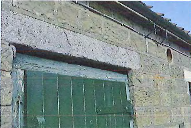
Photo 5: Gaps above doorframe
