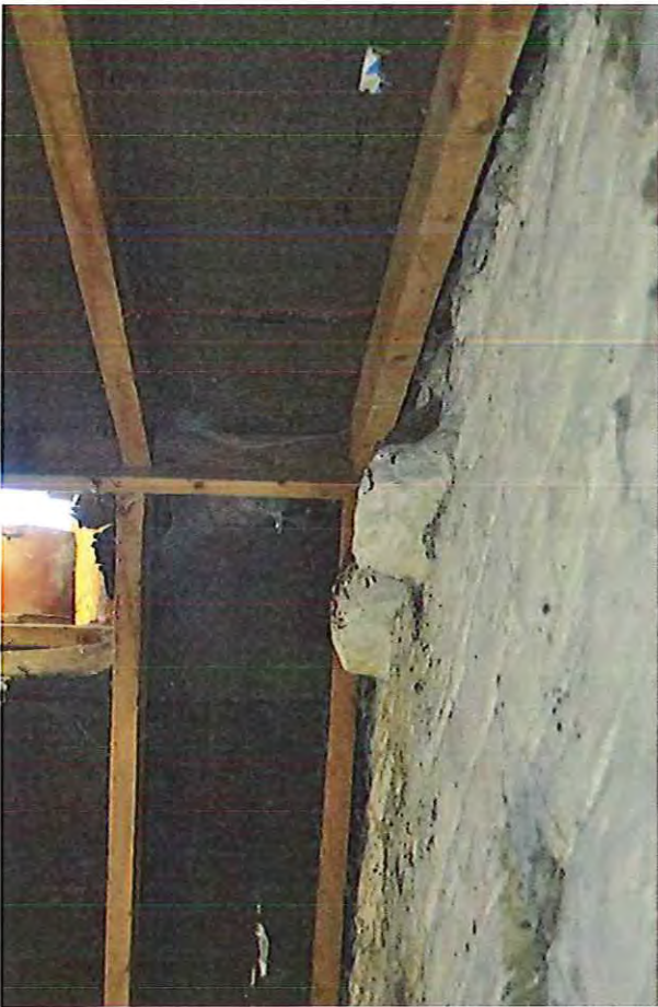
Photo 23: Gaps between rafter and gable end wall.
