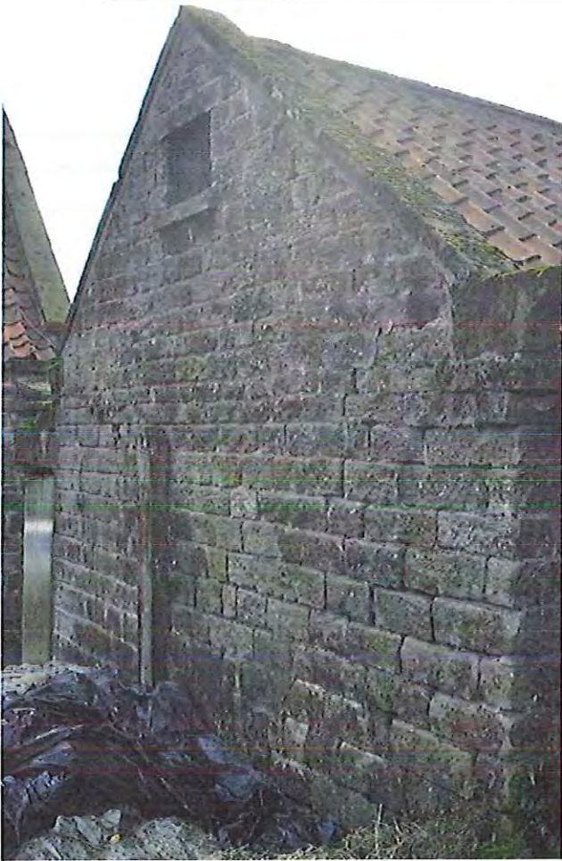
Photo 9: Poor condition of gable end wall
