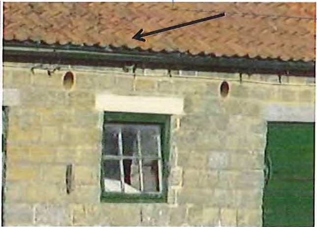
Photo 26: Emergence point form above window.
