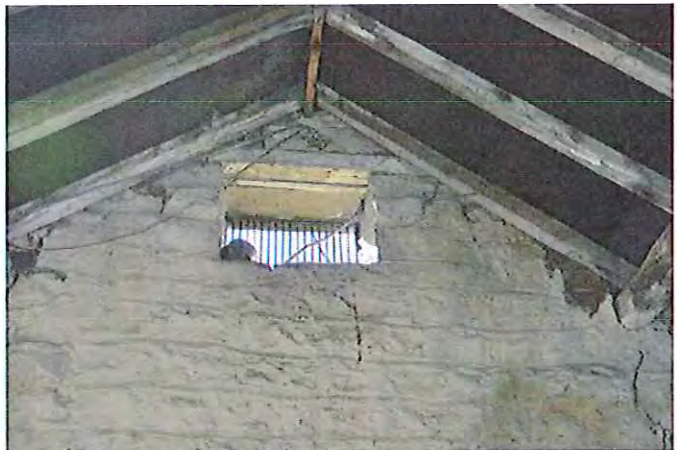
Photo 12: Aperture in gable ed wall with close gapped grill.
