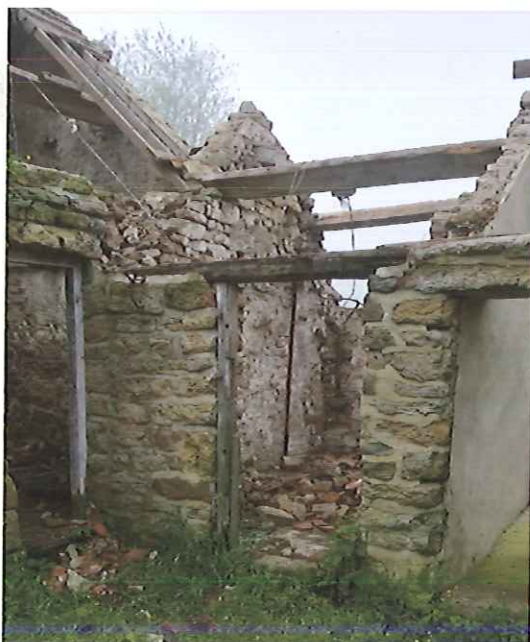
Decayed stone and mortar
