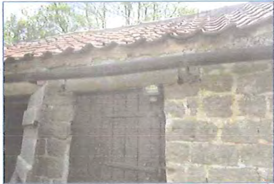
Photo 10 - Crevices around stone door lintel on courtyard elevation.
