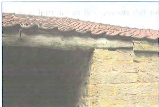
Photo 12 - Crevices around large timber lintel to unit e.
