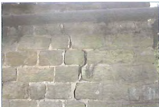
Photo 11 - Masonry crevices within external stone walls (corner of unit e).
