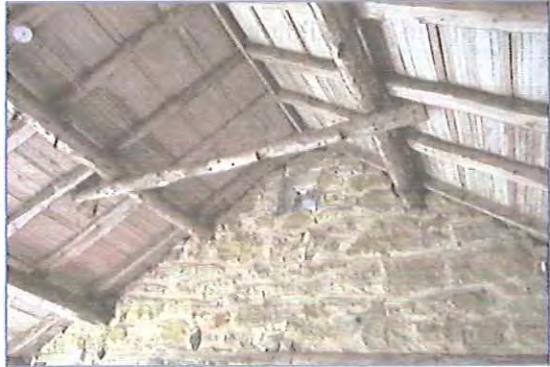
Photo 8 - Roof structure to unit e with timber beam and small gable window used in past by barn owl.
