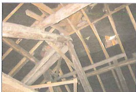
Photo 6 - Cluttered roof structure to unit c.
