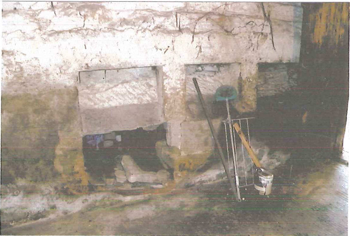
9. Troutsdale Mill. Stone pig feeders in the south wall of Store 3, the old milking parlour.
