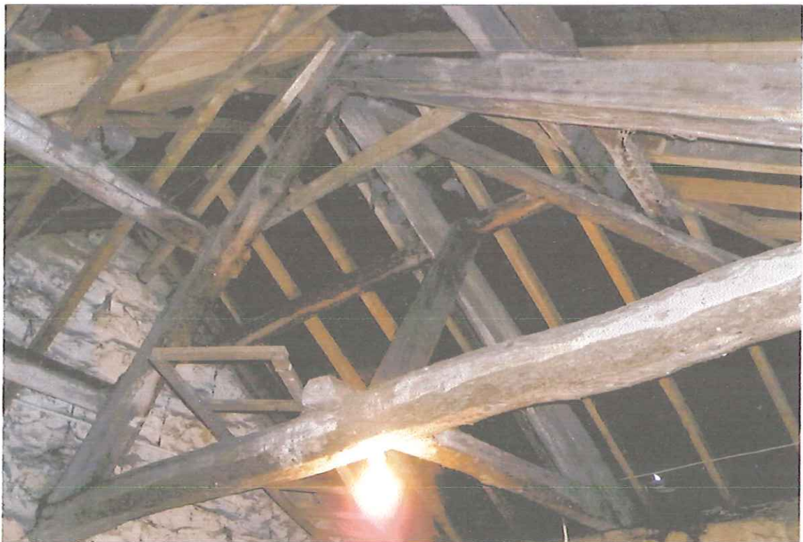
6. Troutsdale Mill. Collared roof truss in the half-hipped roof over Store 3, the old milking parlour.
