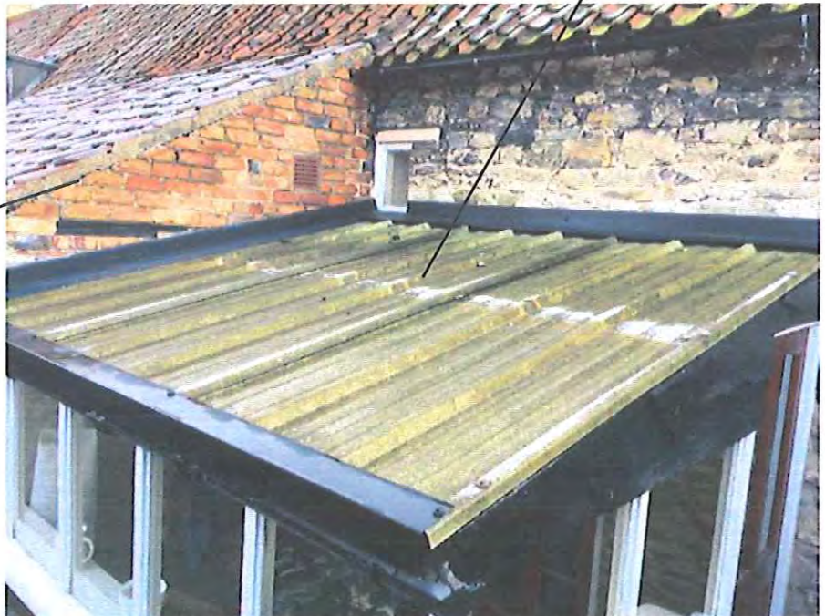
replacement pantiled roof to be raised to same level as existing roof over kitchen
