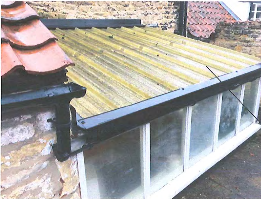
existing profiled fibreglass roof to be removed and replaced with natural clay pantiles
