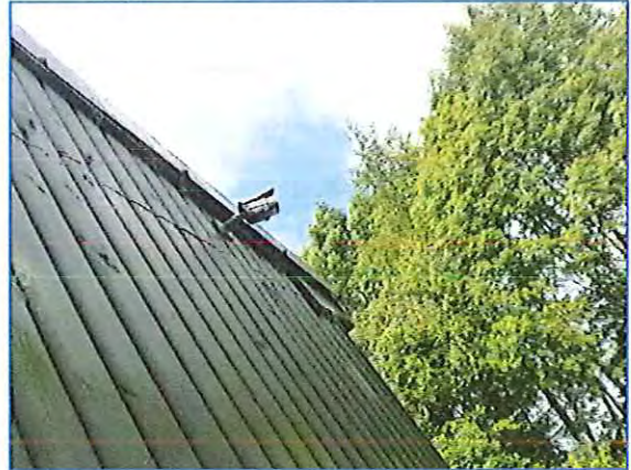
Photo 5: Gap behind fascia on north gable.
