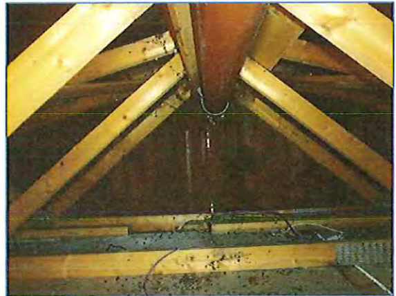
Photo 7: Bat droppings below central beam near south gable..
