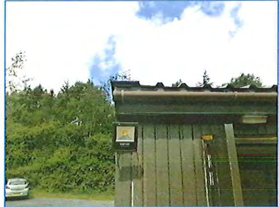
Photo 3: Gap under roof at eaves.
