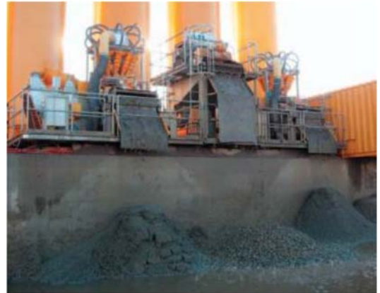
Figure 2: Typical Desanding Unit
