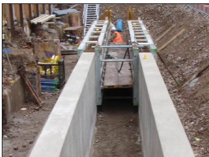
Figure 4: Access platform between vertical shutters.
