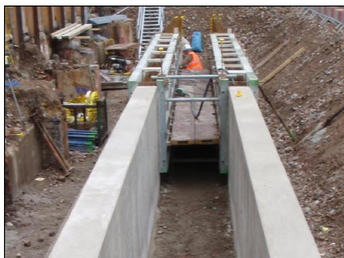
Figure 4: Access platform between vertical shutters.
