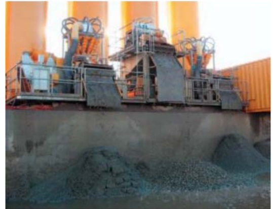
Figure 2: Typical Desanding Unit
