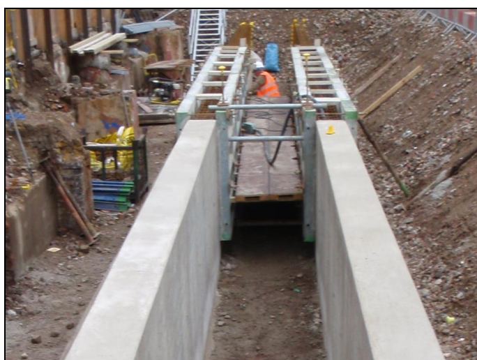
Figure 4: Access platform between vertical shutters.
