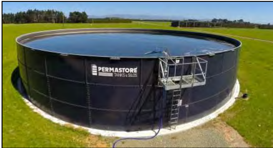
Figure 4: Photograph of typical storage tank
