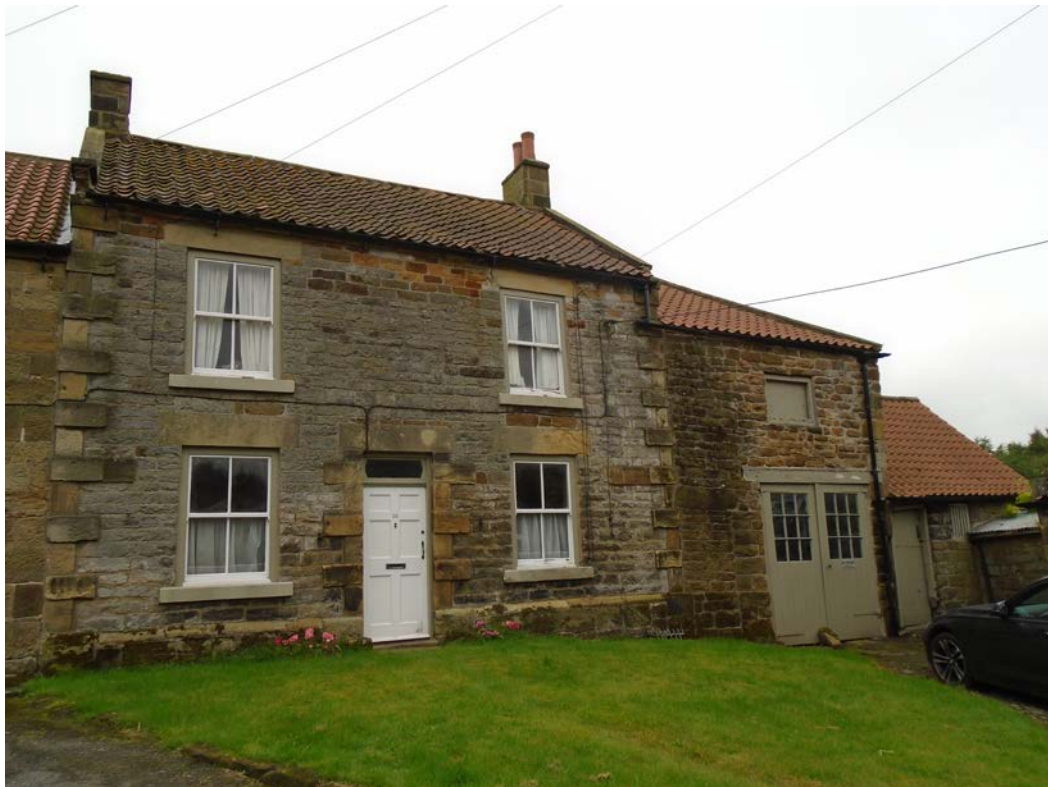
Figure 2 View looking south-west towards principal elevation of No. 10 South End. Note first-floor stonework and ground-floor blocked doorway of coach house.
