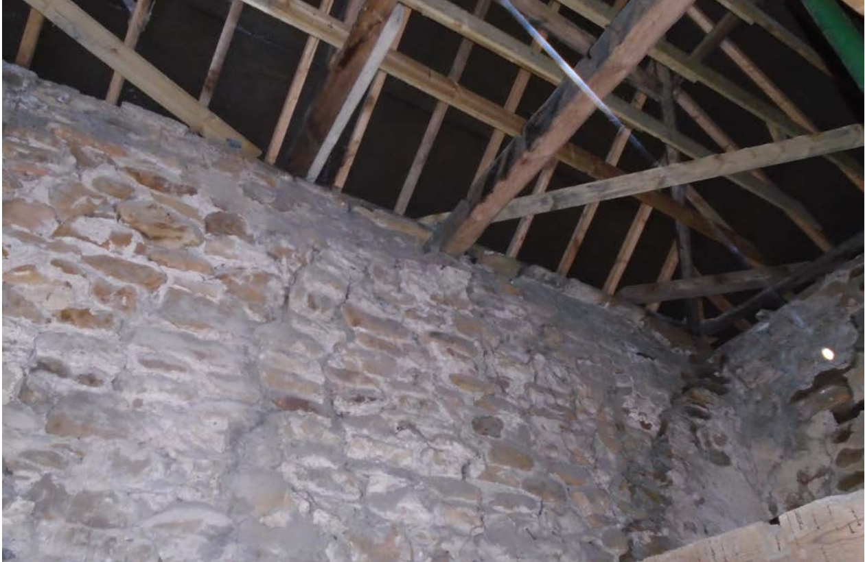
Figure 11 Cracked wall and renewed roof timbers
