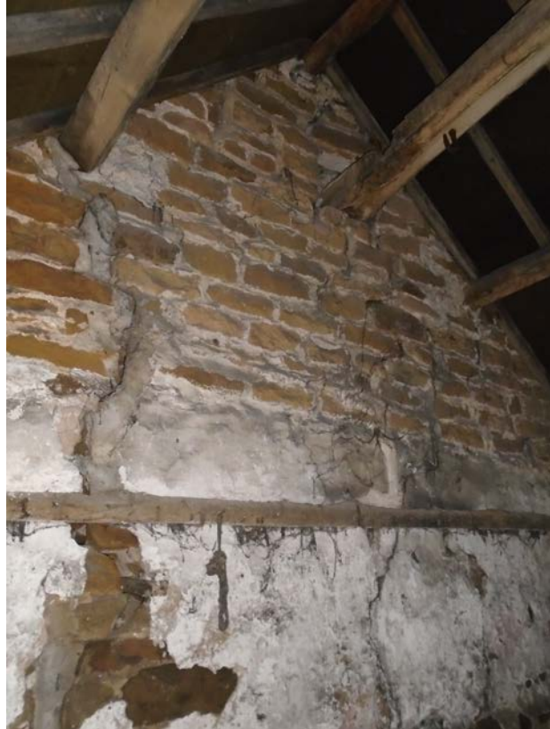
Figure 13 Outside wall of coach house, now south wall of stable. Note large crack in stonework.
