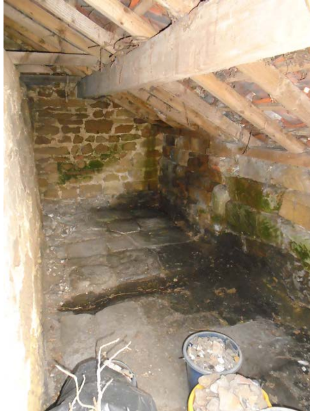
Figure 9 Right room of pigsty
