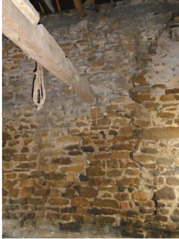
Figure 12 Interior north wall of coach house, note crack in stone wall
