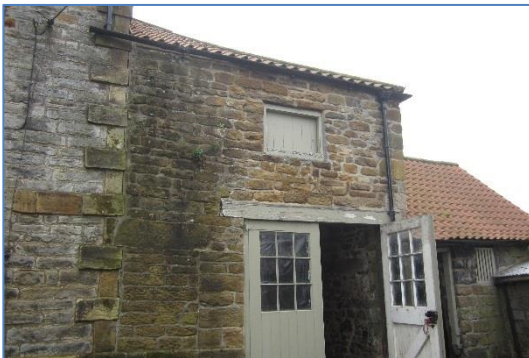
Photo 1: Block A – Cart house and Block B Front Outhouse to west (righthand single storey building)
