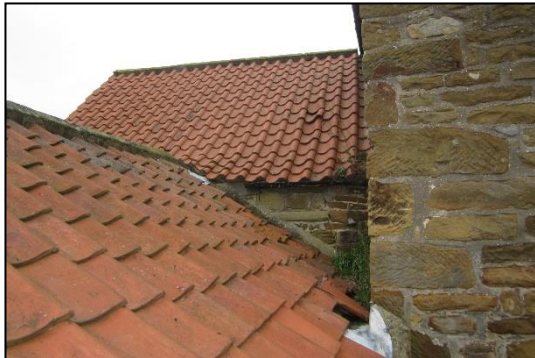
Photo 3: Loose tile on rear of Block B
