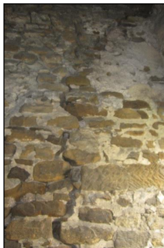
Photo 8: Large masonry crack in Block A
