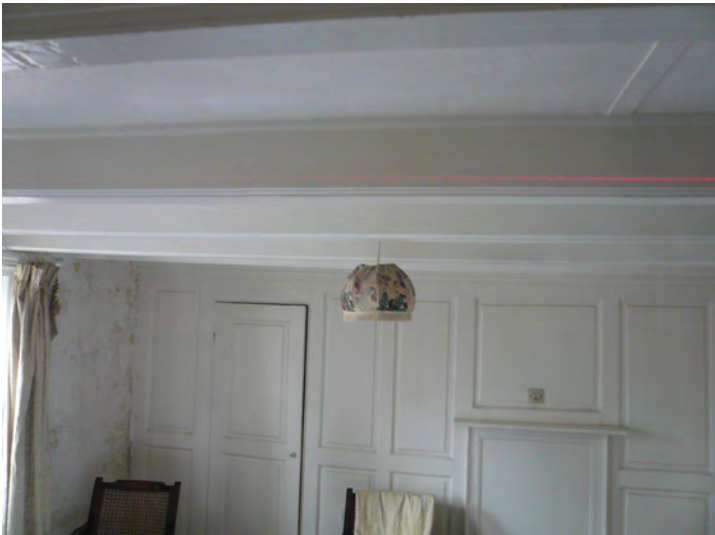
Photograph 3. Second Floor joists. Deflection approximately 40mm.
