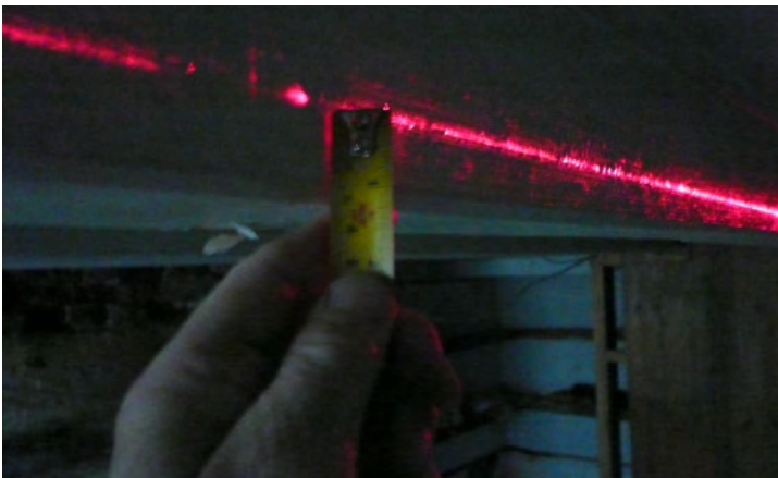
Photograph 1. Shows deflection of GFL joists approx 30mm.
