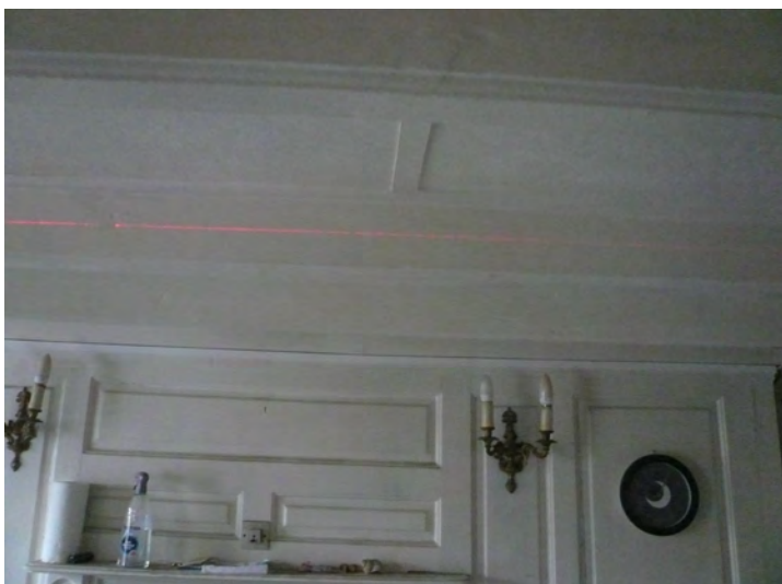
Photograph 2. Shows deflection of FFL joists of approximately 70mm.
