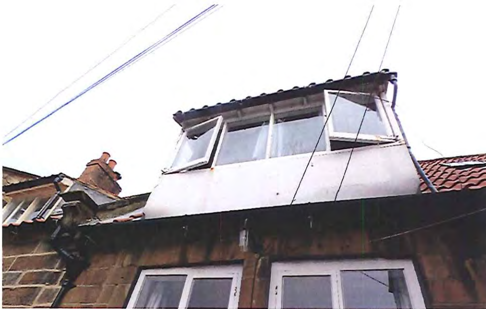
W11 – Replace existing Dorma single glazed timber windows with slim double glazed windows
