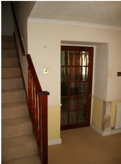
Photos 18a and 18b - Existing doors and frames removed and replaced with ledge and brace solid oak doors (RM06).
