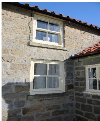
Photo 17 - Existing window W16 to be replaced on an exact like for like basis excl internal horn detail (RM06).
