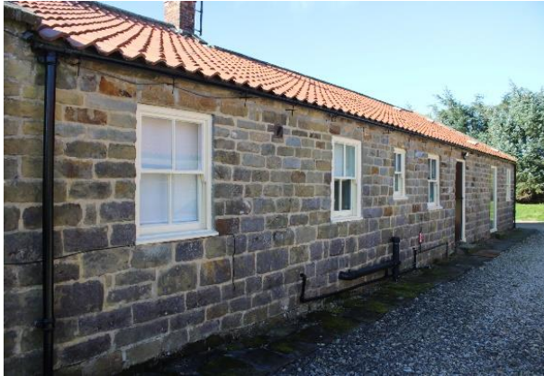
Photo 13 – Existing single glazed window W07 to be replaced with timber sliding sash double glazed window (RM05).
