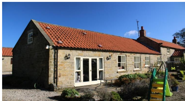
Photo 31 - Head height increased to accommodate new floor level with reclaimed timber lintel. New external timber doors and frame installed with reclaimed timber mullion (labelled D5) (RM14).
