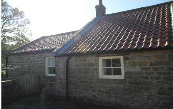
Photo 9 - Existing single glazed window W08 to be upgraded and double glazing inserted (RM03).
