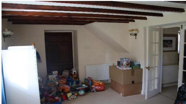
Photo 10 – Opening (white door) reduced and new ledge and brace solid oak door & frame installed (RM04).
