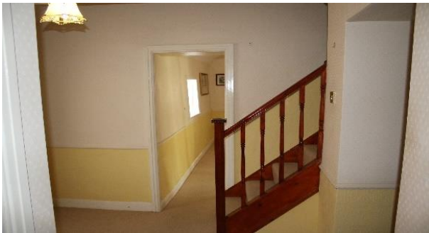
Photo 14 – Lower 2 steps of staircase to be modified (RM05).
