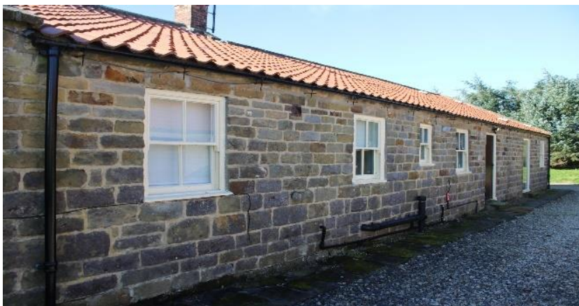
Photo 22 - Existing single glazed window W05 to be replaced with new timber sliding sash double glazed window (RM08).
