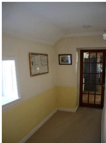
Photo 8 - Glass door to RM02 to be removed and replaced with new ledge and brace solid oak door.
