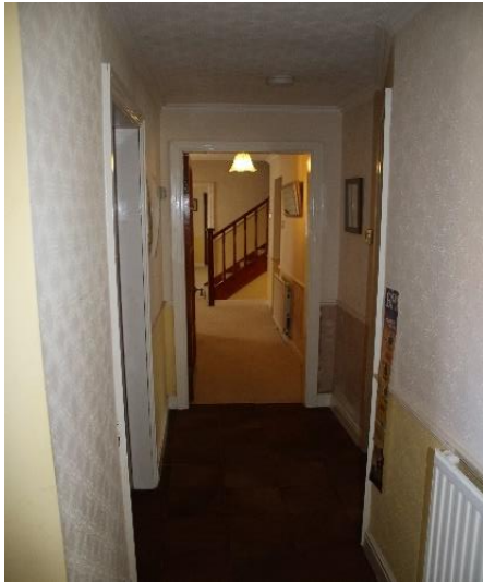
Photo 23 – Reconfiguration of spaces off passage, ledge and brace solid oak doors to internal rooms (RM09).
