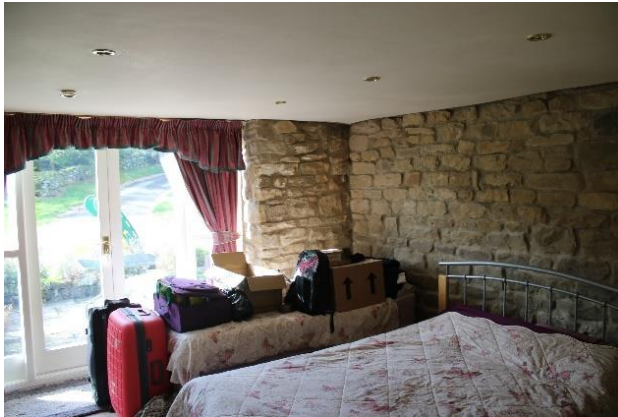
Photos 32a and 32b – Low ceiling to be taken down and vaulted ceiling inserted (RM14).
