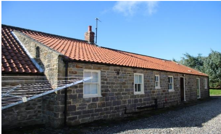
Photo 27 - Existing single glazed window W04 to be replaced with new timber sliding sash double glazed window together with rear porch addition (RM11).
