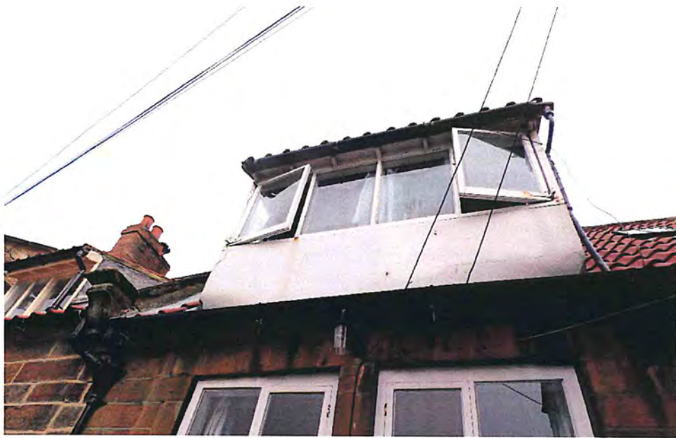
W11 – Replace existing Dormer single glazed timber windows with slim double glazed windows
