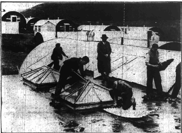
PREPARING THEIR TRAINING CENTRE.—Some of the first men at the Allerston Instructional Centre erecting huts in the camp, to be officially opened shortly.
