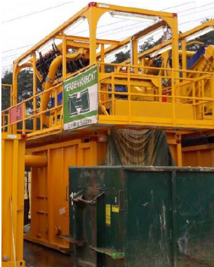
Extractive materials filtration (de-sander/de-silter)
