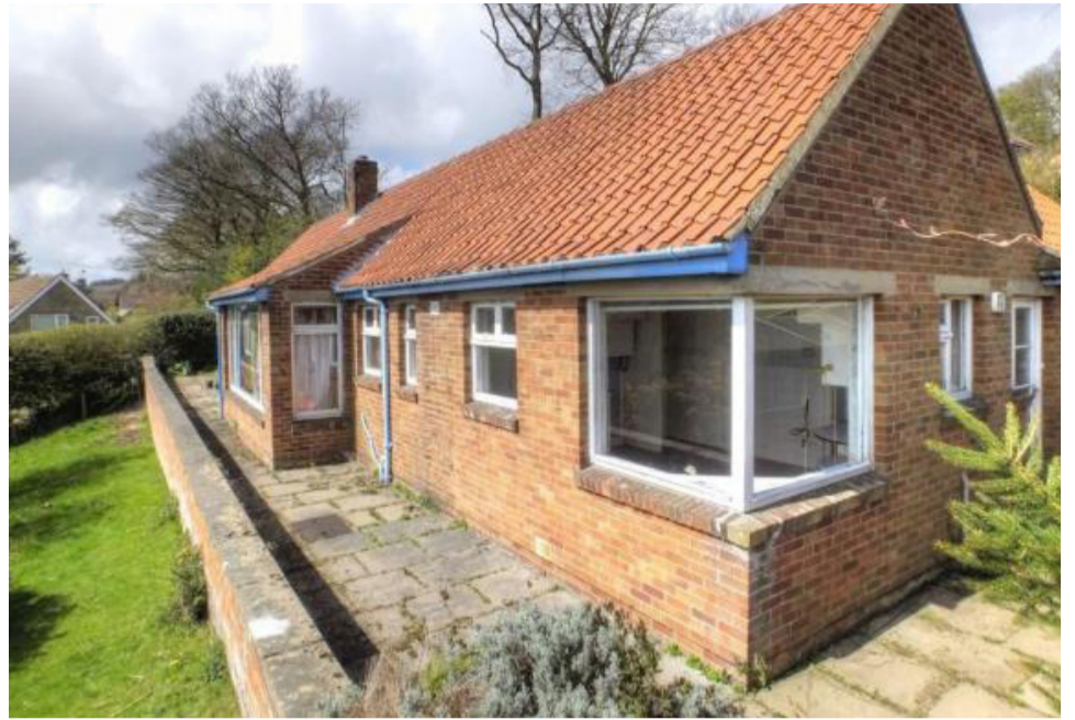
Existing dwelling - East/South elevation: Existing corner windows to be removed as part of new fenestration arrangement.
