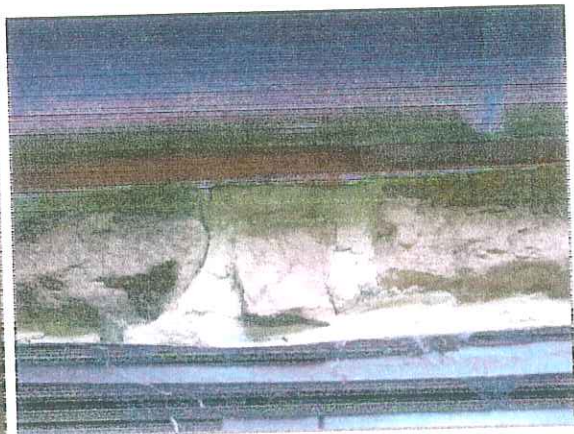
Fig. 7 Small gap at eaves at rear of bungalow
