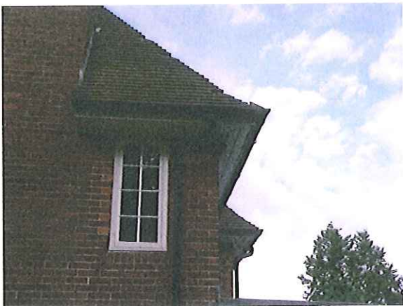
gaps adjacent to windows.
