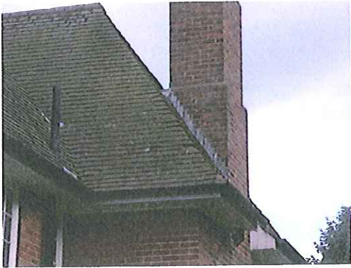
gaps in hip tiles and soffit boards.
