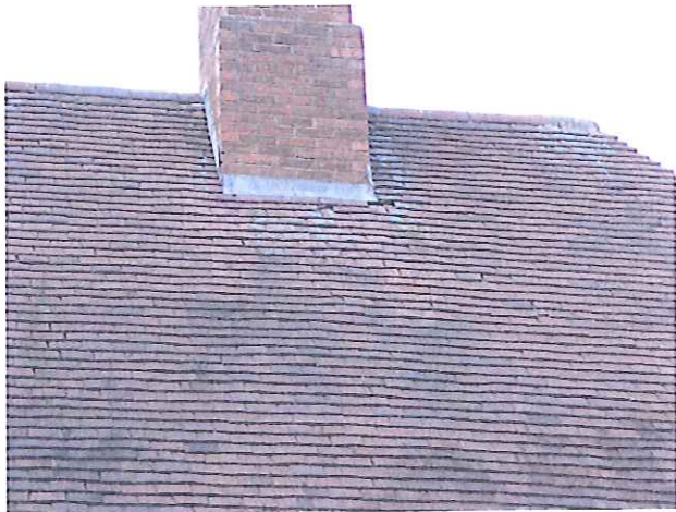
gaps under flashings.
