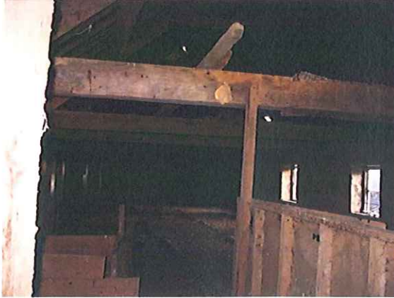
Photo 2 Bitumastic lined felt in compartments 2, 11, 10.
