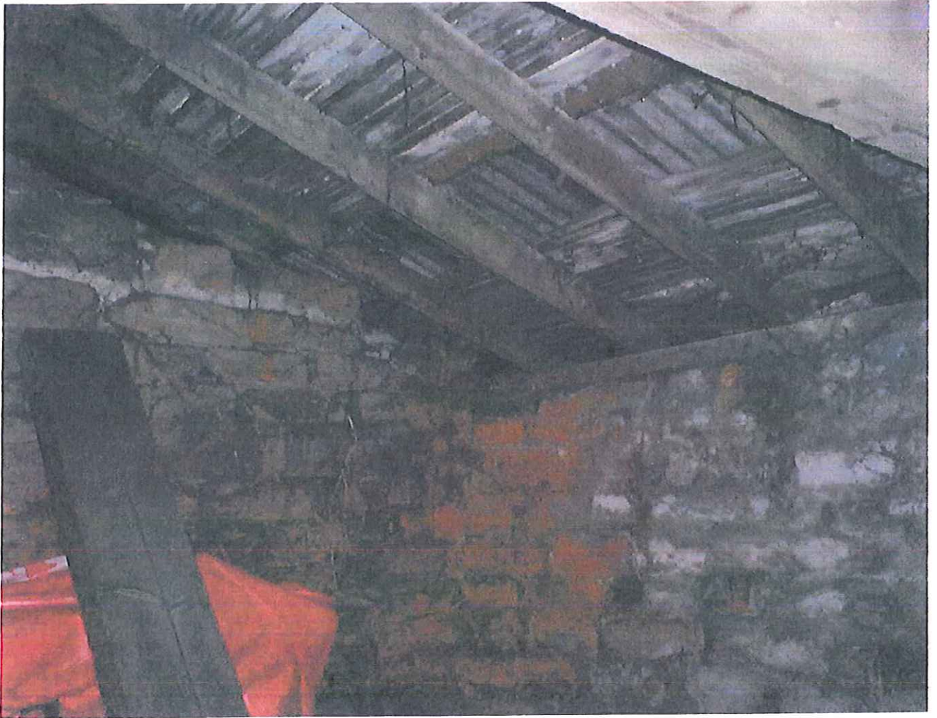
Appendix 1: Detail of North facing wall and roof taken from within the building.
