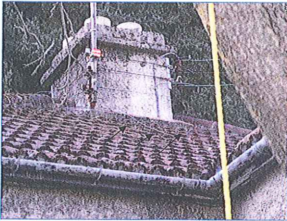
Photo 7. Gaps between roof tiles
