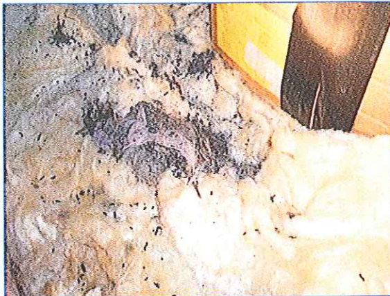
Photo 5. Collection of droppings close to chimney breast
