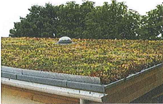
Sedum Green roof to reduce visual impact and blend in with surroundings
