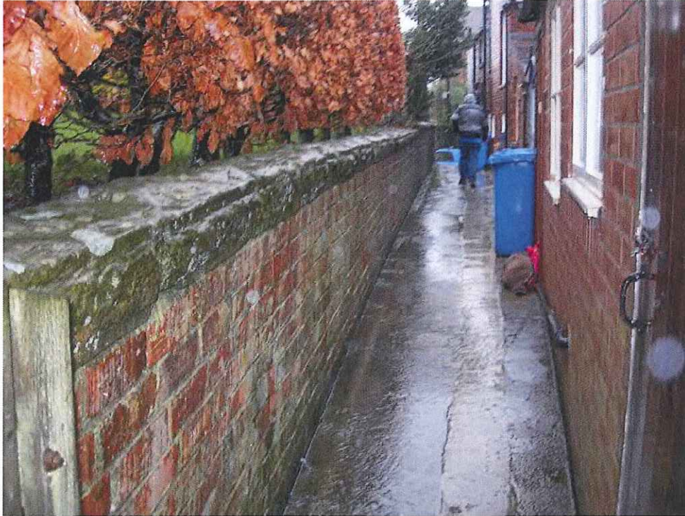
Water flooding out of the bottom of the boundary wall. Notice sandbags at base of doors opposite.
